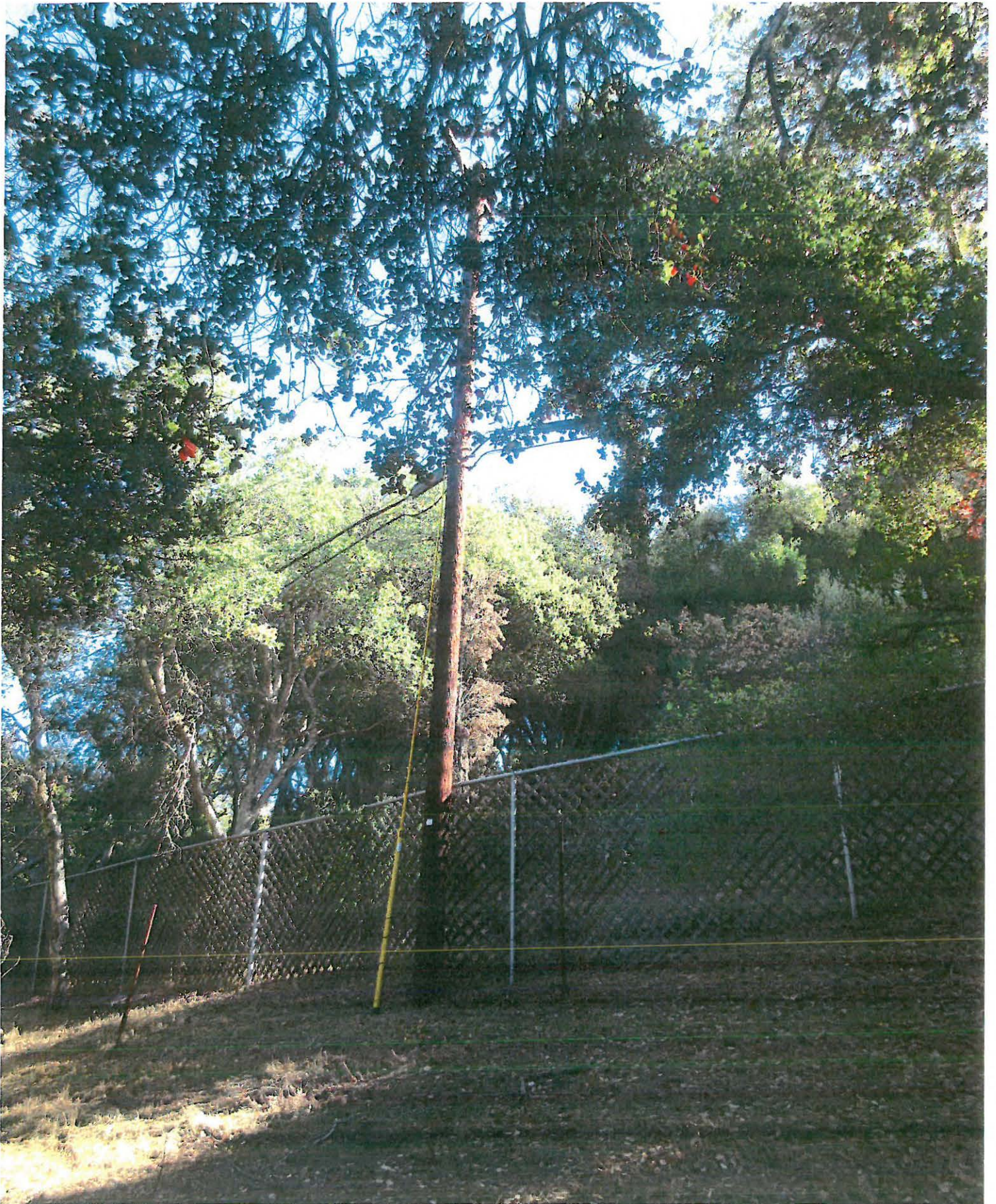
Dist.49 Deteriorated Pole L / E
