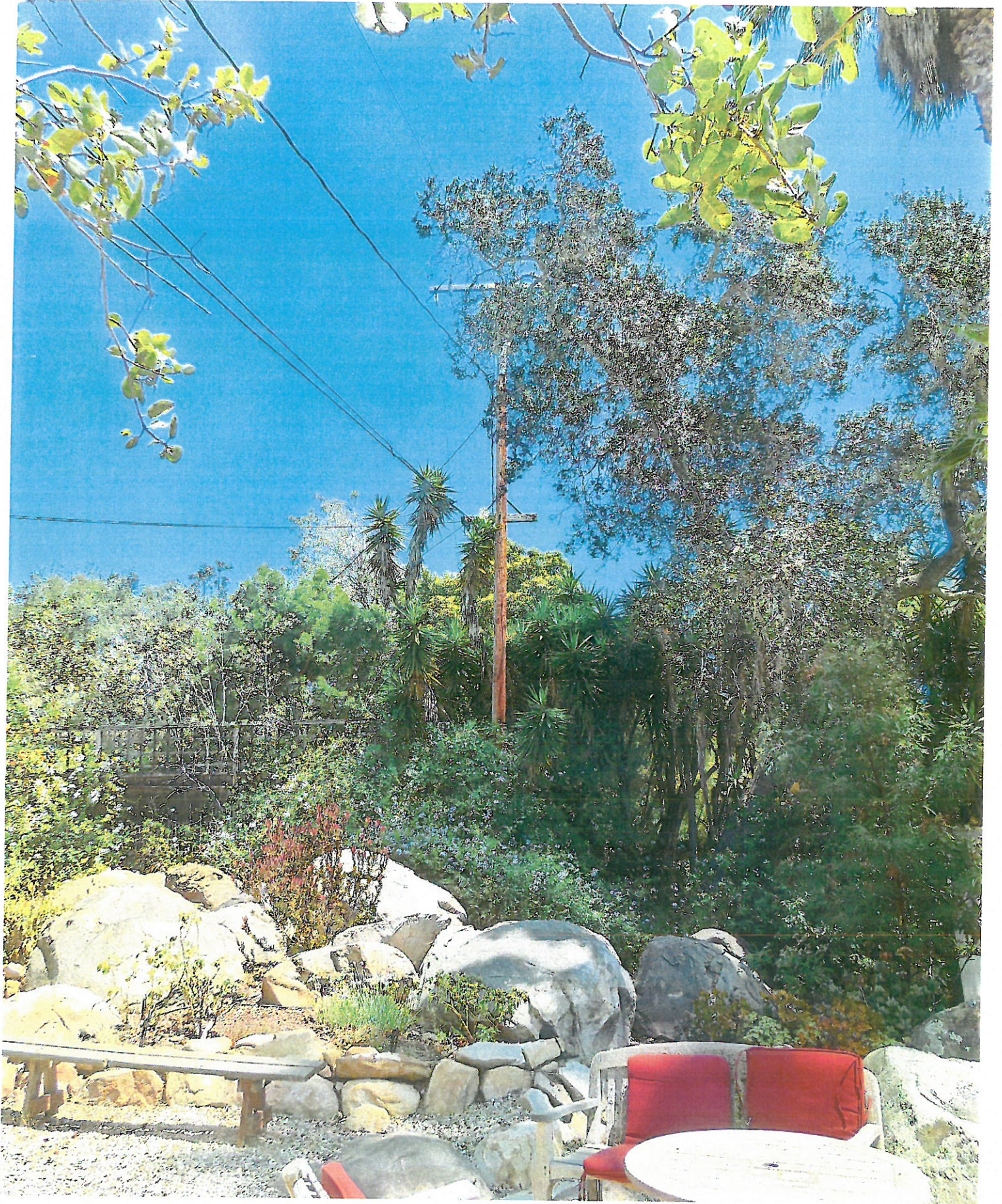
Dist. 49Deteriorated Pole L / E
