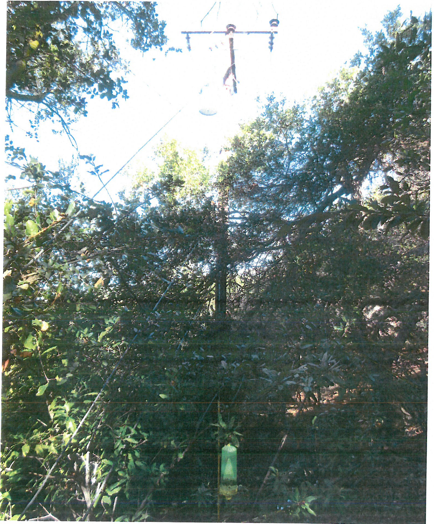
Dist.49 Deteriorated Pole L / N
