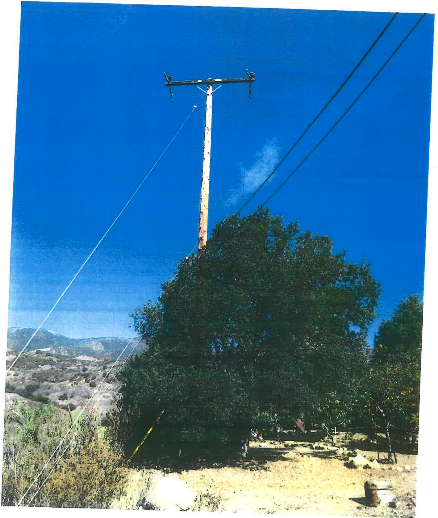
Dist.49 Deteriorated Pole L / N
