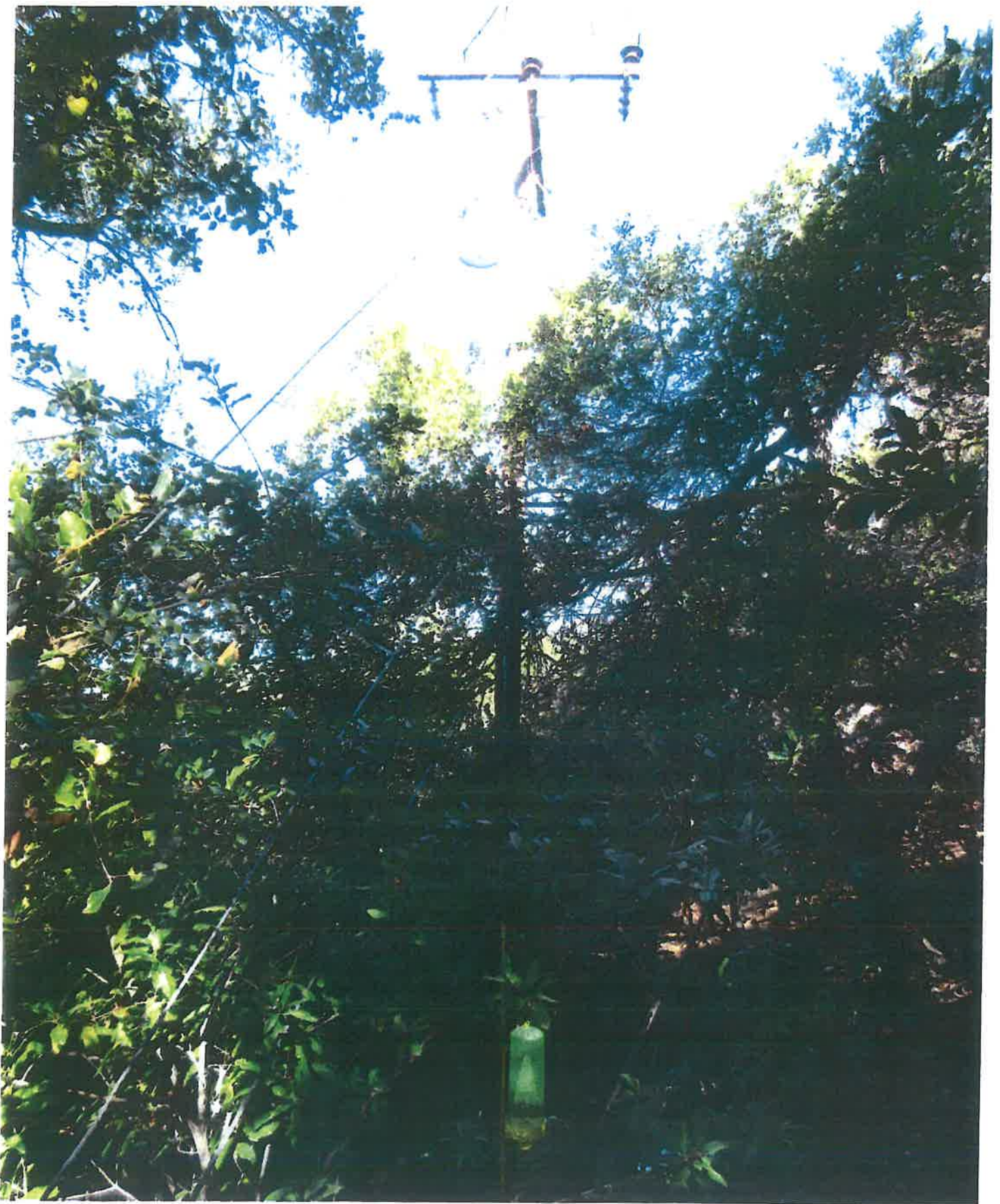
Dist.49 Deteriorated Pole L / N
