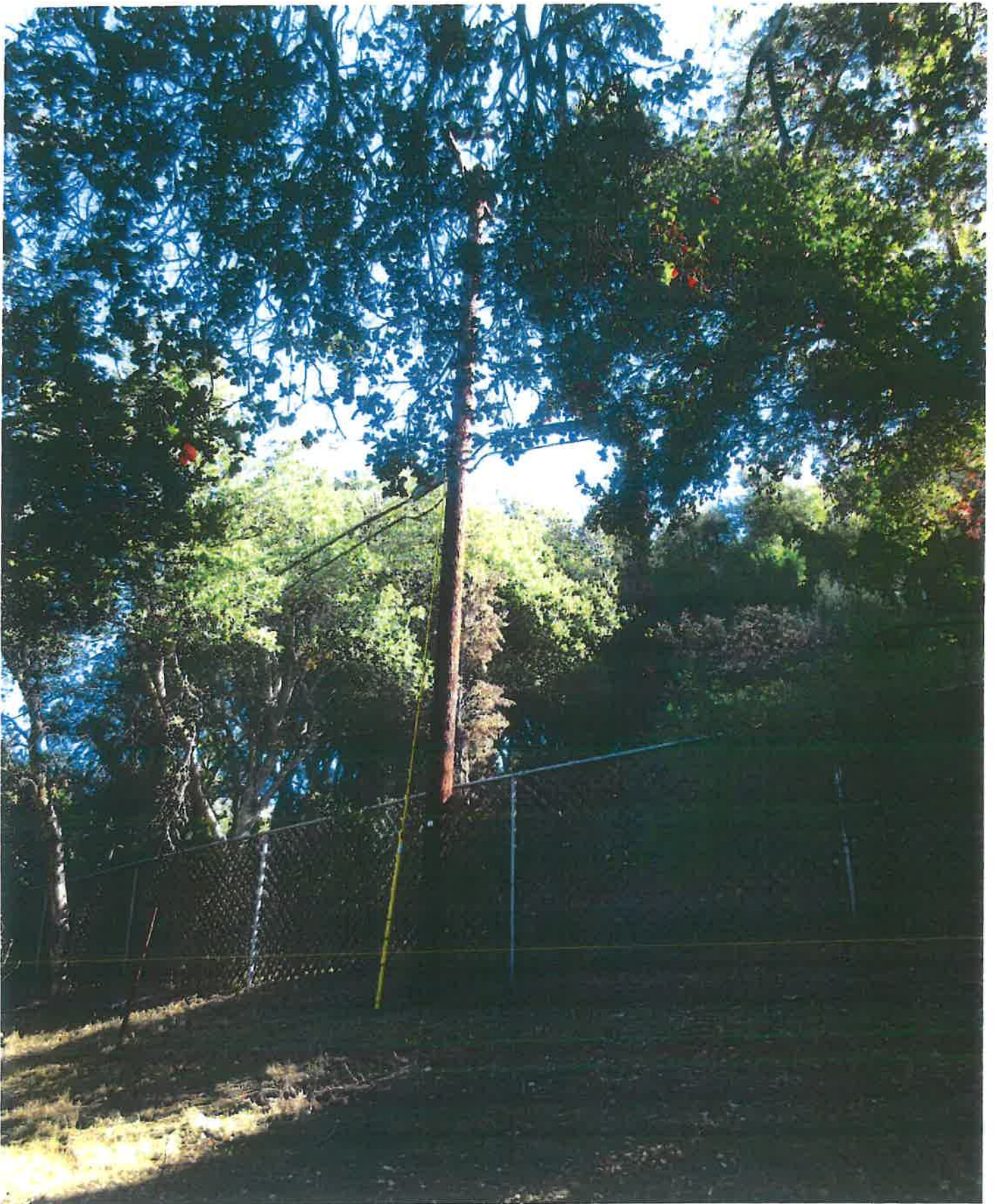
Dist.49 Deteriorated Pole L / E
