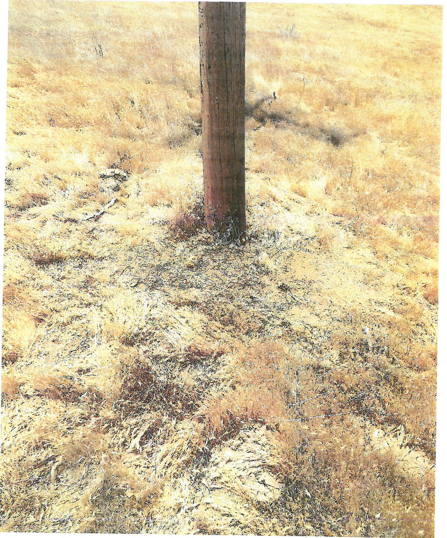
Dist. 36 Deteriorated Pole L / N
