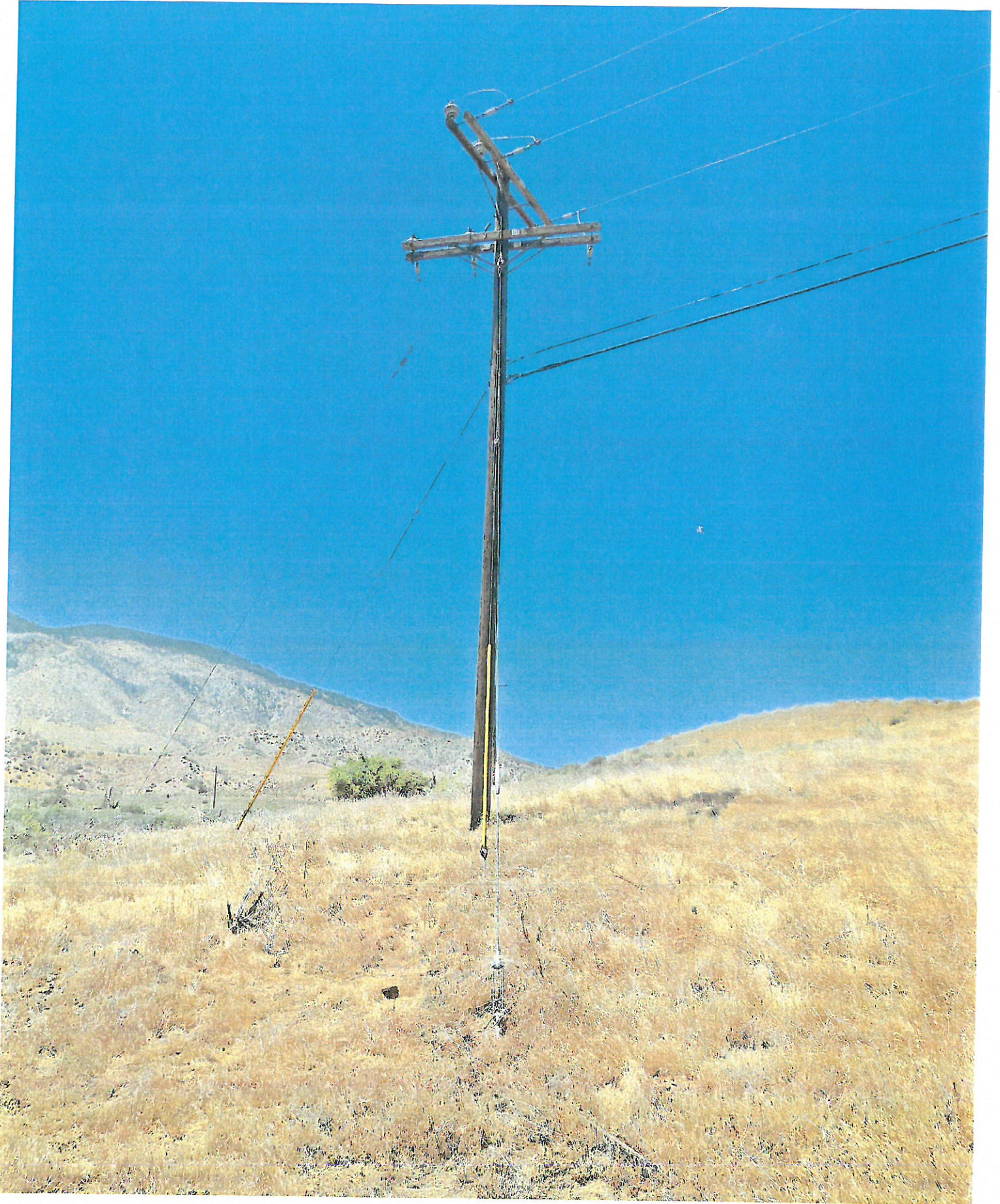
Dist. 36 Deteriorated Pole L / W
