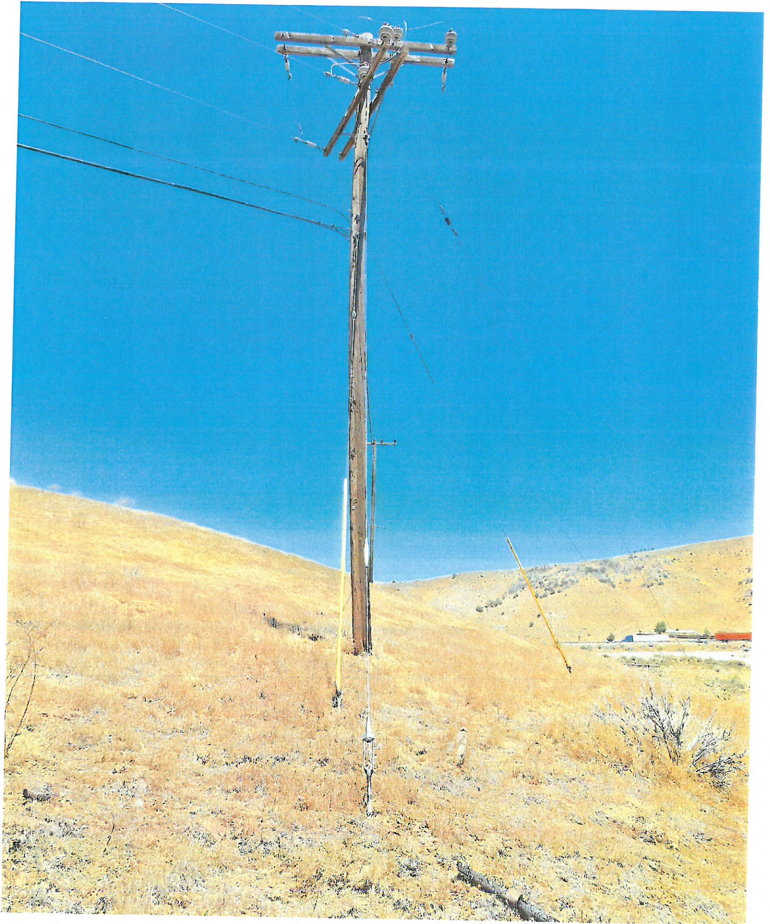
Dist. 36 Deteriorated Pole L / N
