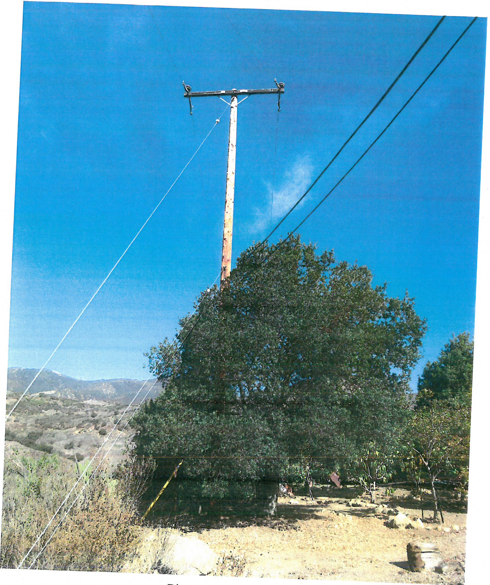
Dist.49 Deteriorated Pole L / N
