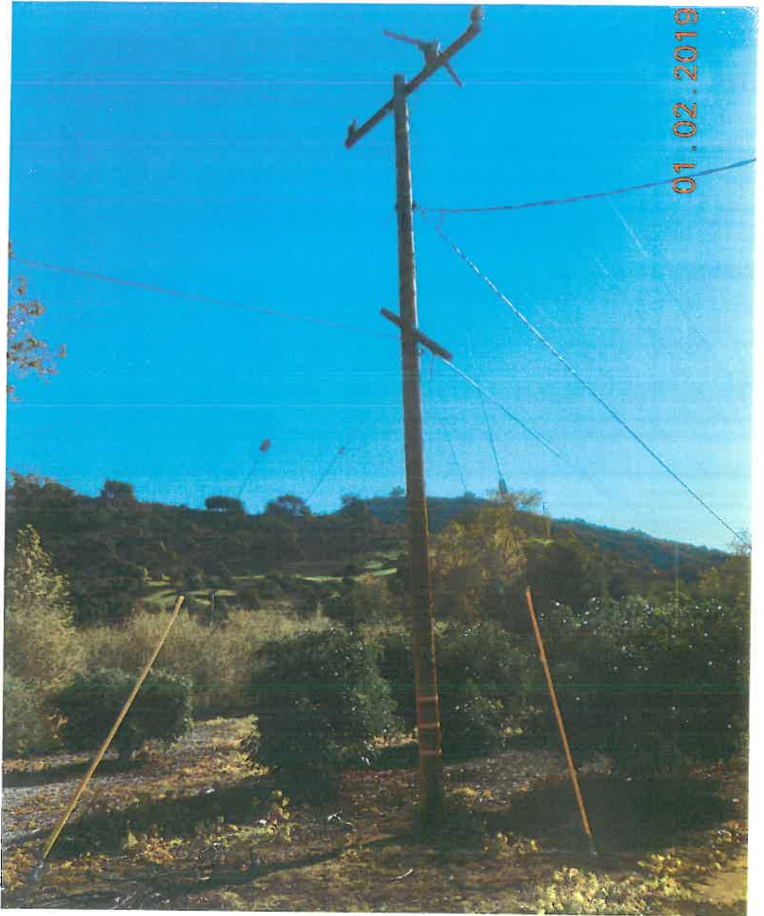
Dist.49 Deteriorated Pole L / E
