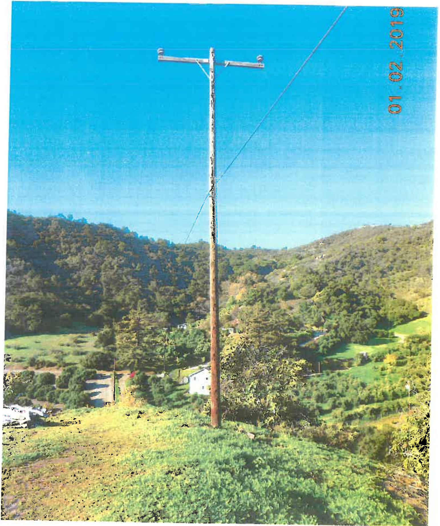
Dist.49 Deteriorated Pole L / SW
