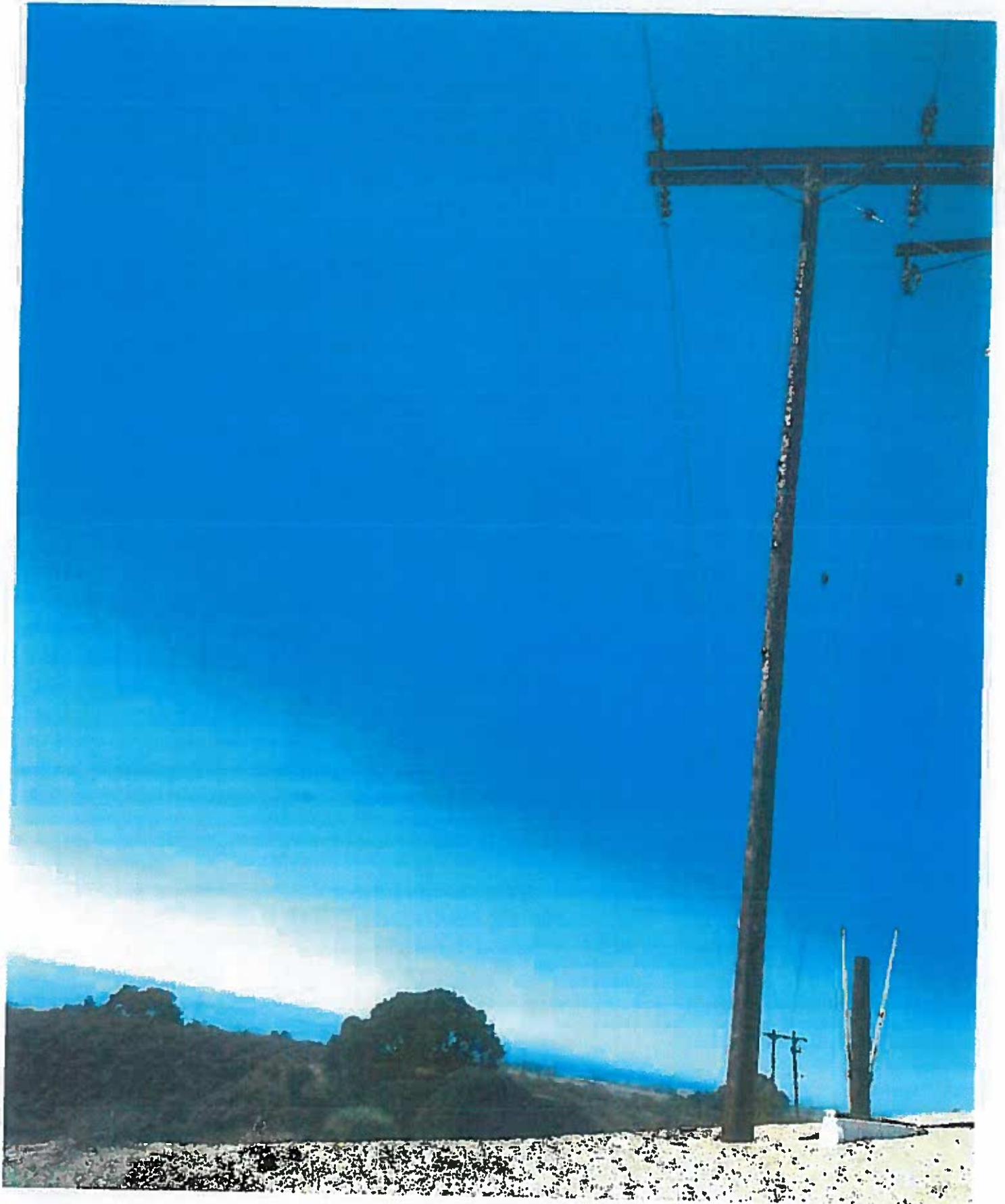
Dist.49 Deteriorated Pole L / W
