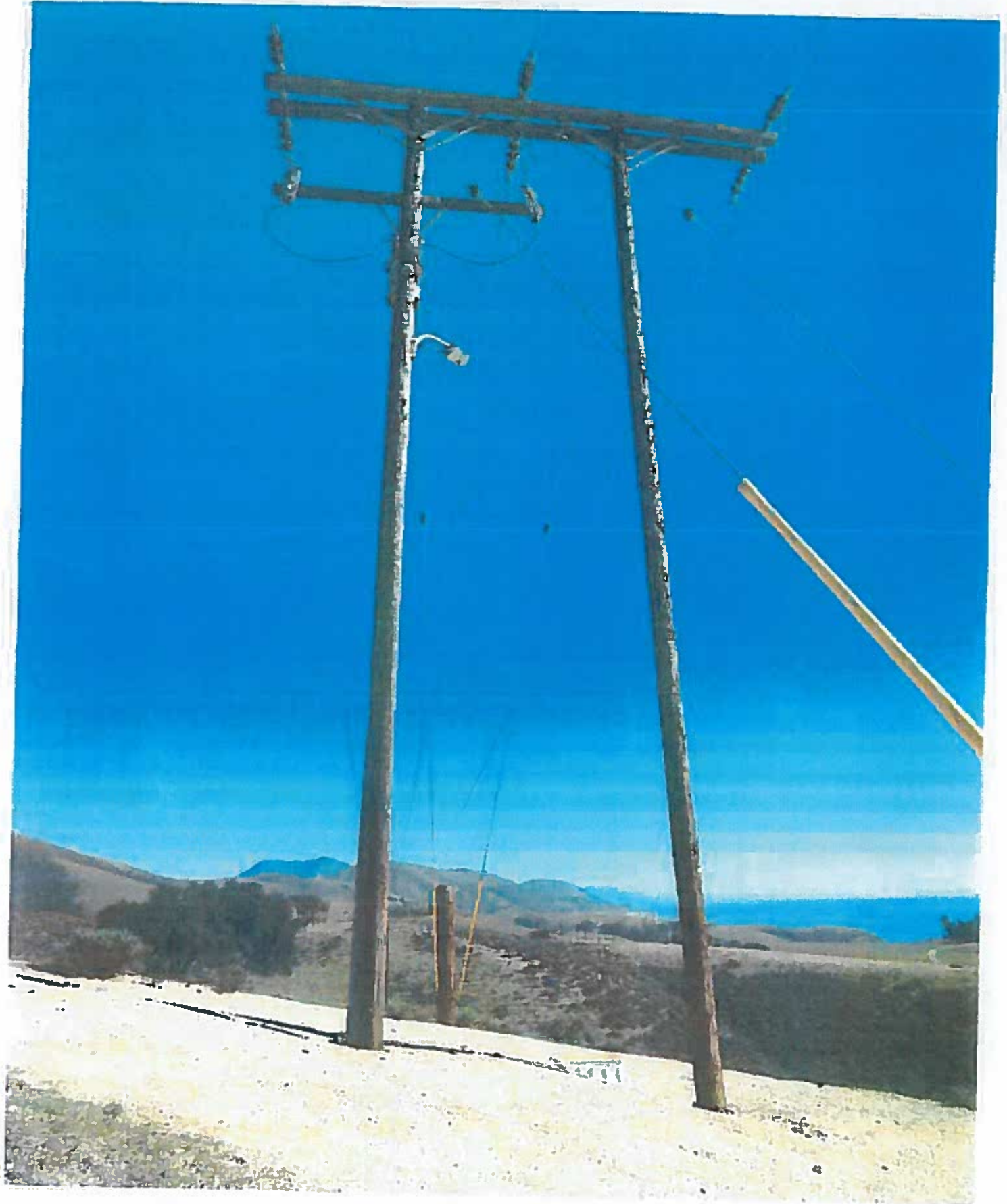
Dist.49 Deteriorated Pole L / E
