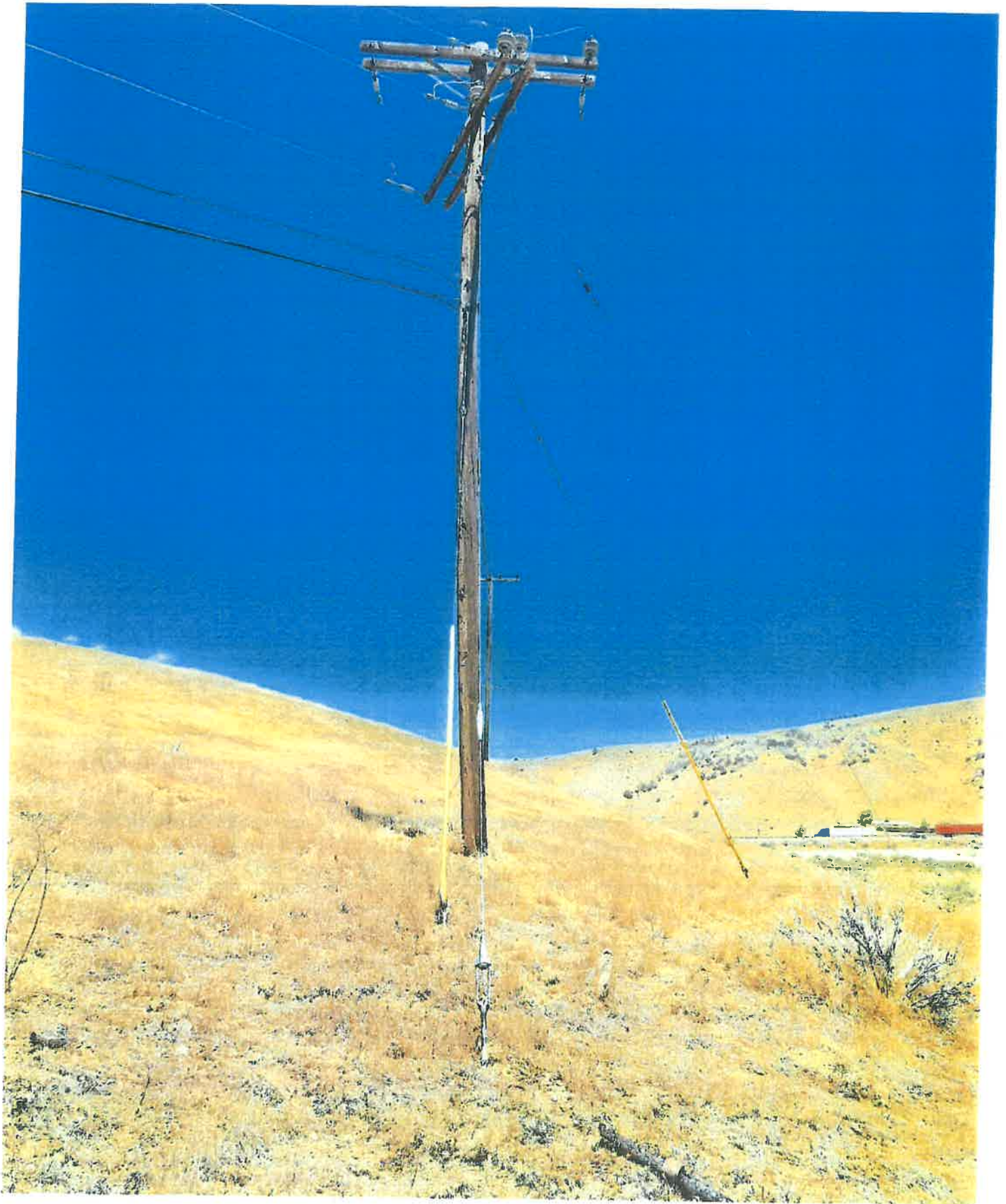
Dist. 36 Deteriorated Pole L / N
