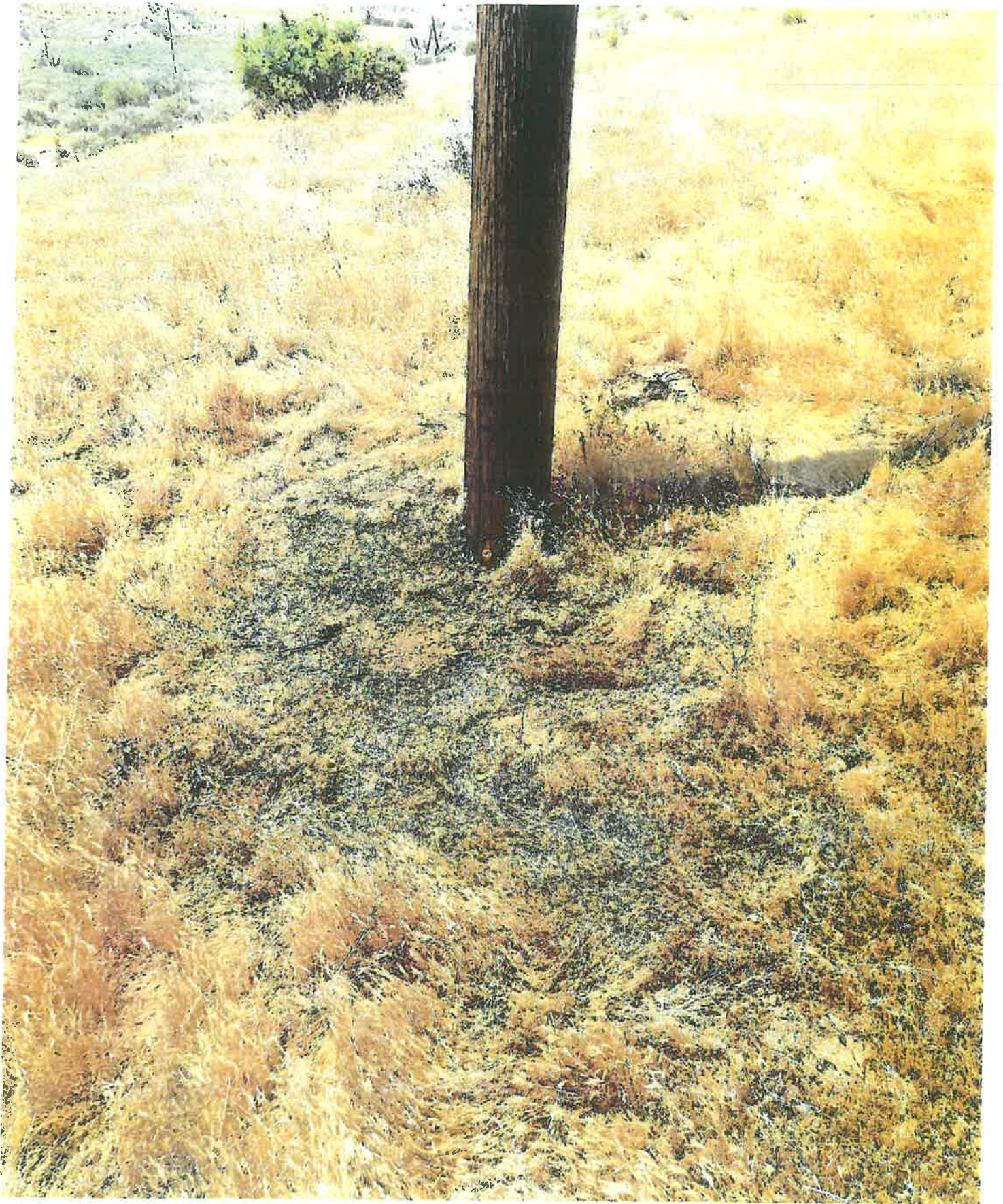
Dist. 36 Deteriorated Pole L / W
