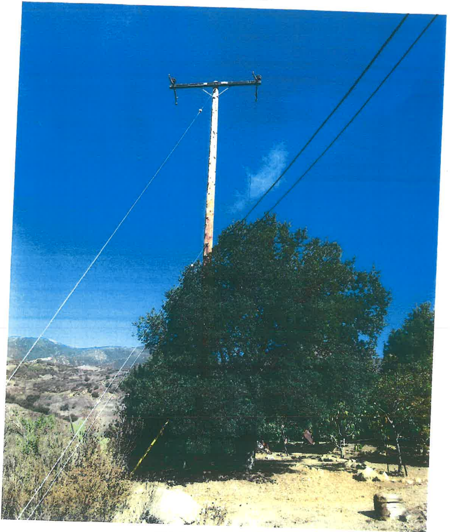
Dist.49 Deteriorated Pole L / N
