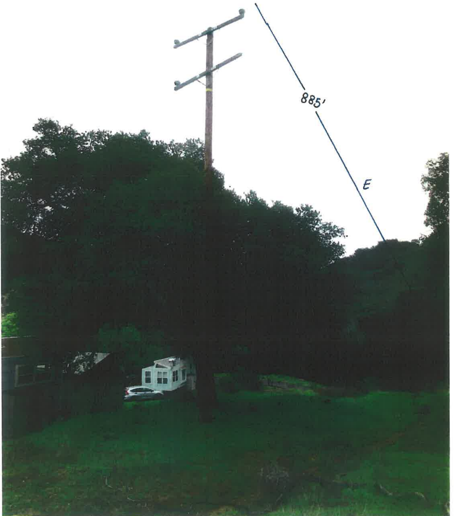
Dist.49 Deteriorated Pole L / NE
