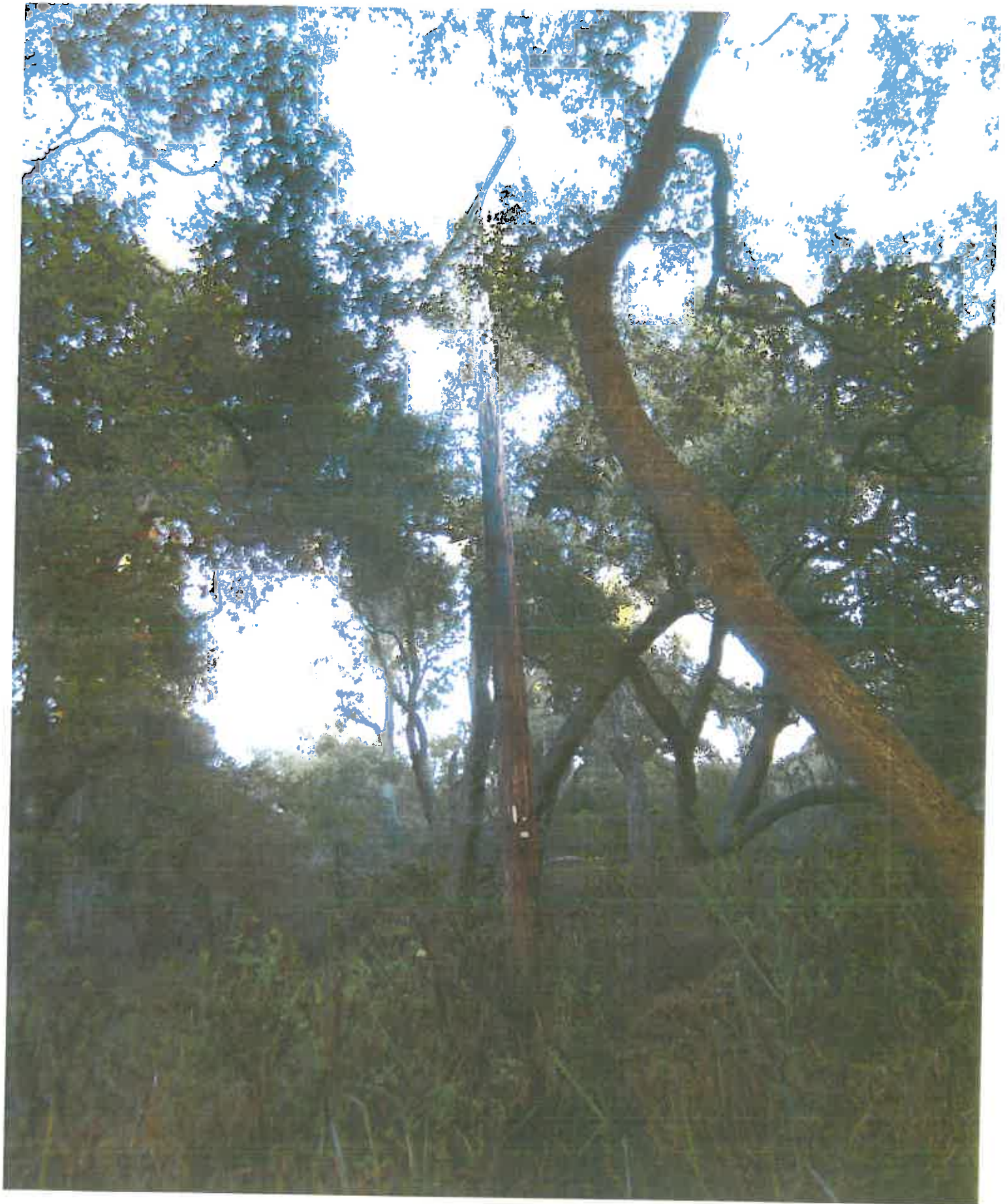
Dist. 49 Deteriorated Pole L / SE
