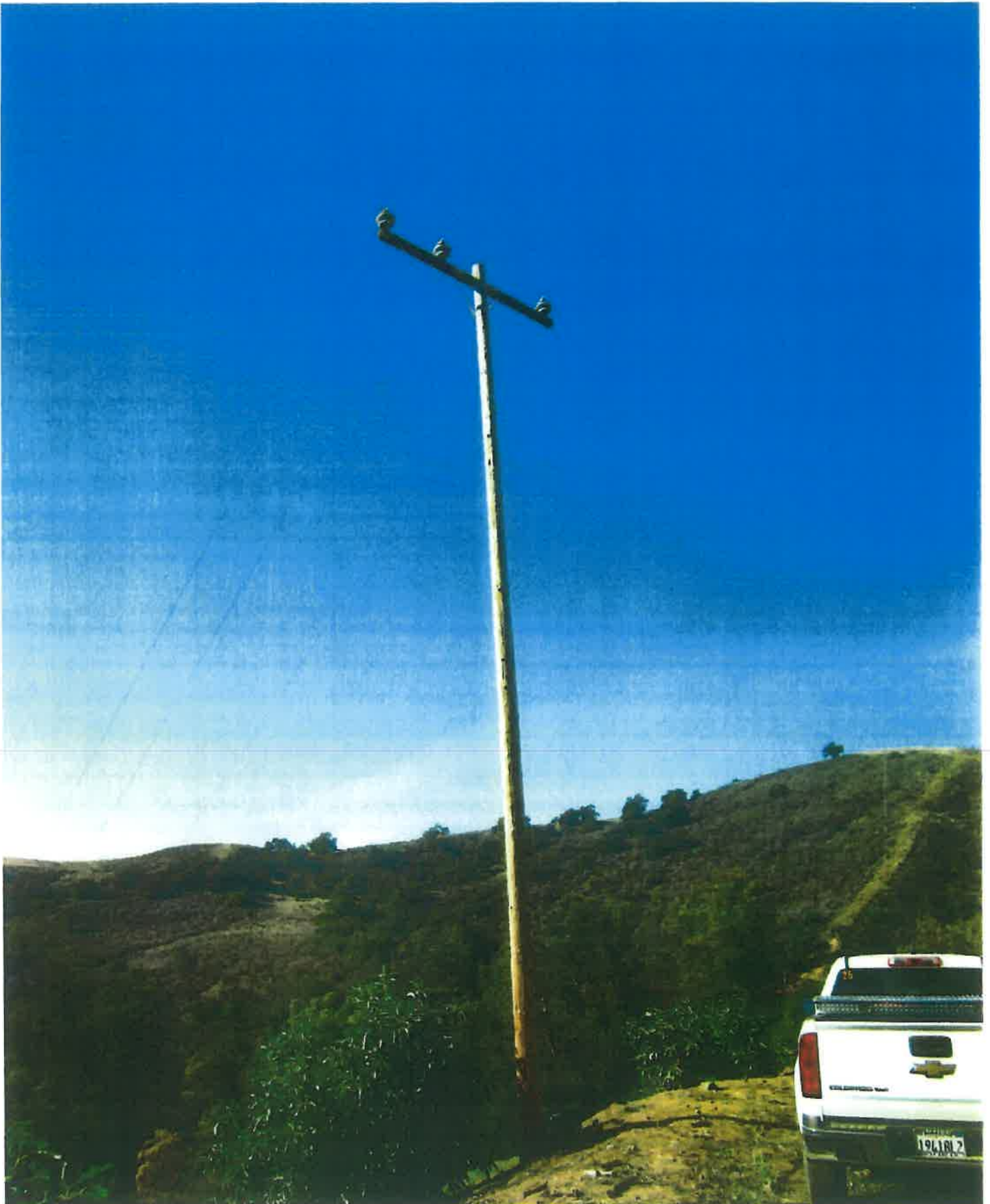
Dist. 49 Deteriorated Pole L / W
