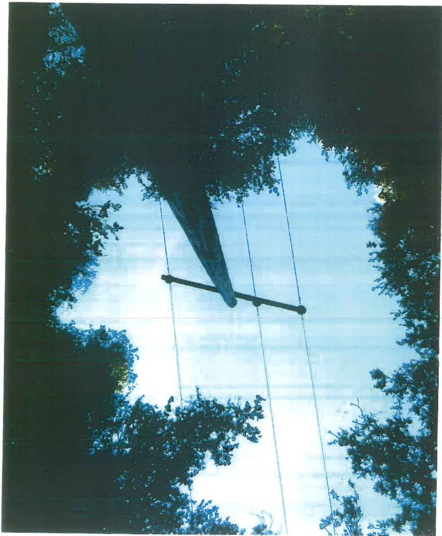
Dist. 49 Deteriorated Pole L / NE
