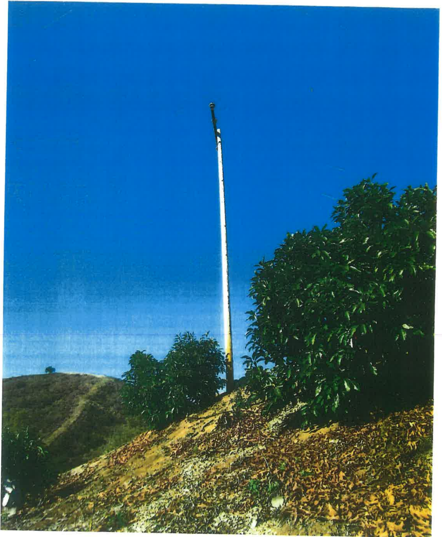
Dist. 49 Deteriorated Pole L / NW
