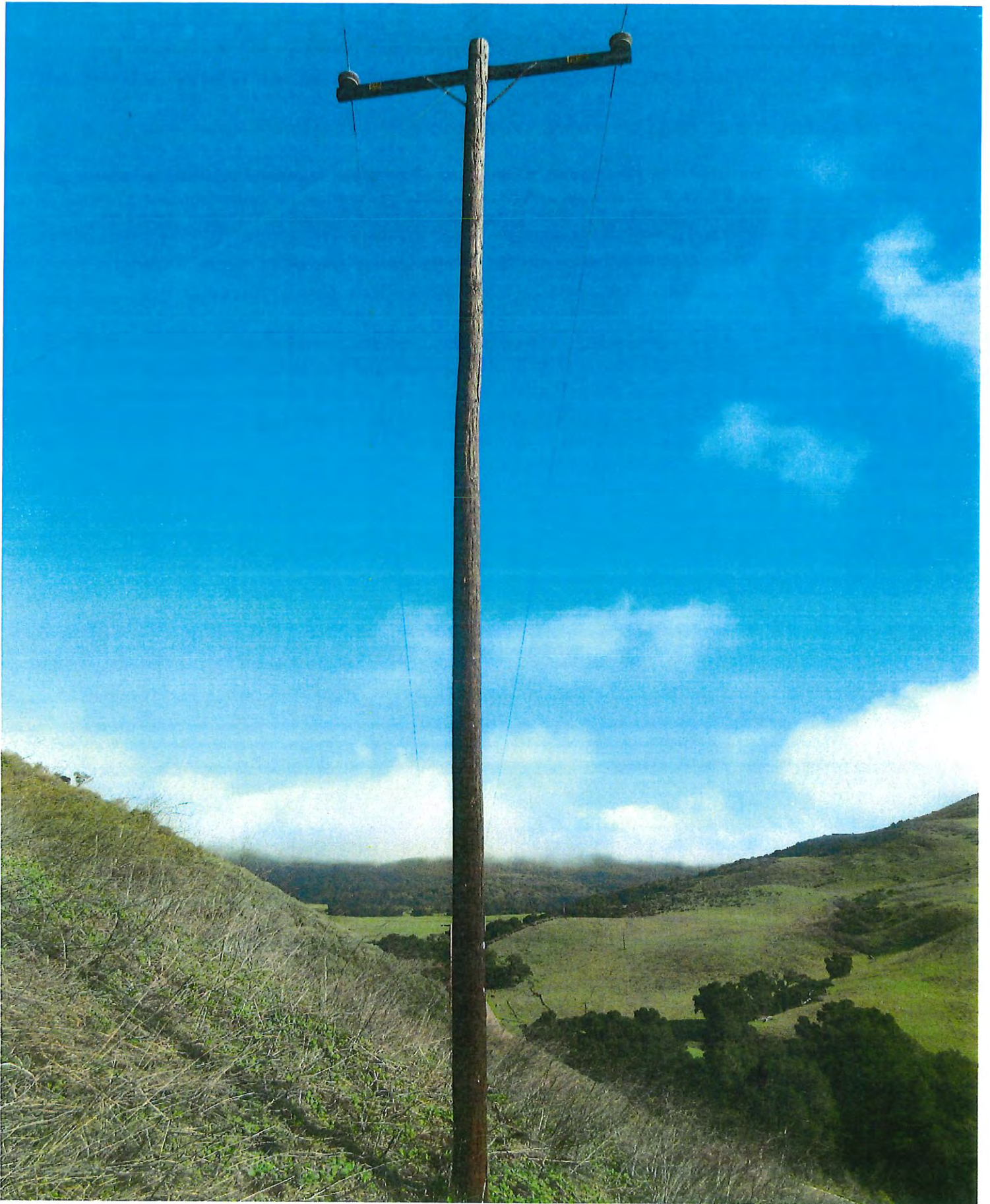
Dist.49 Deteriorated Pole L / N
