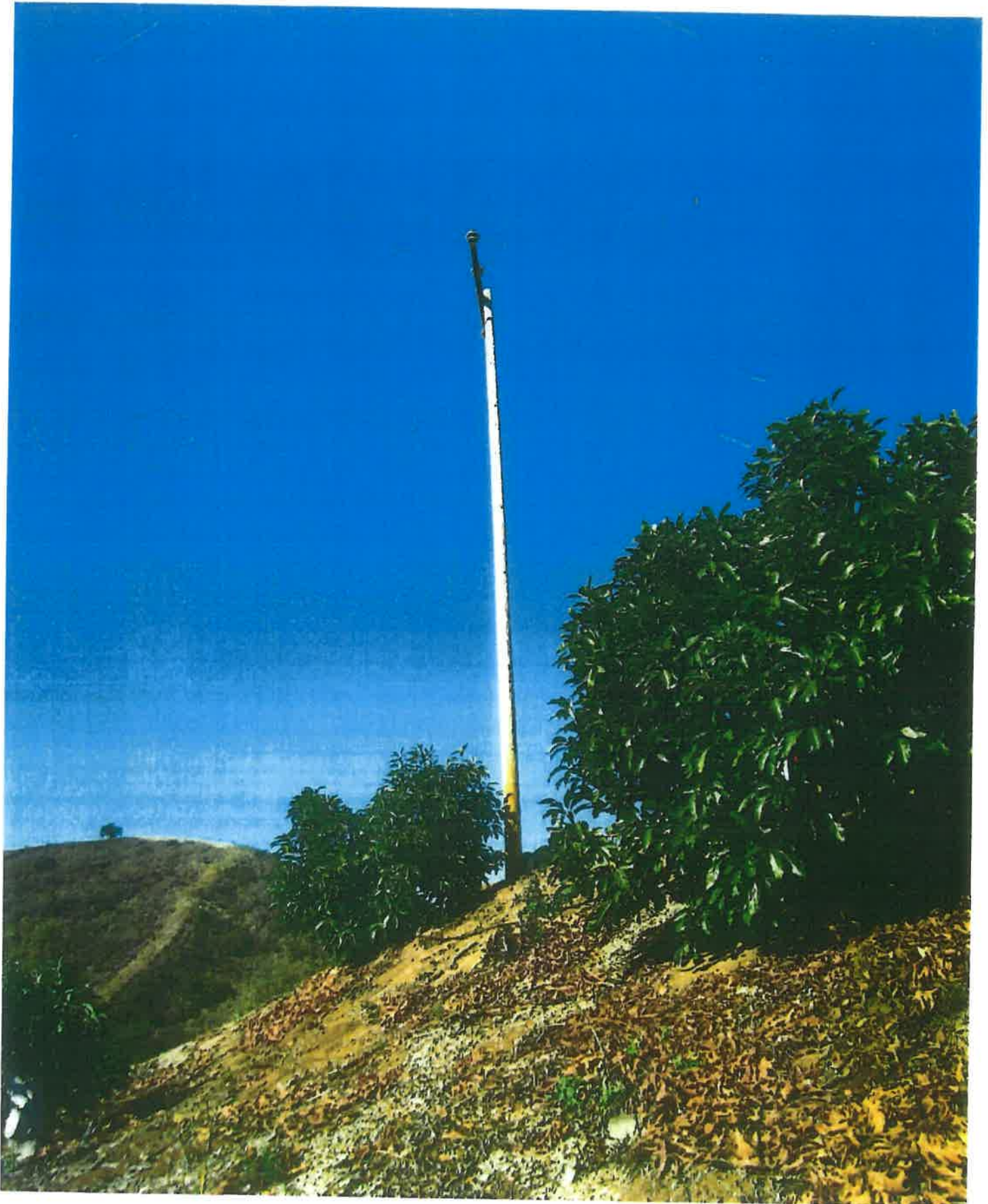
Dist. 49 Deteriorated Pole L / NW
