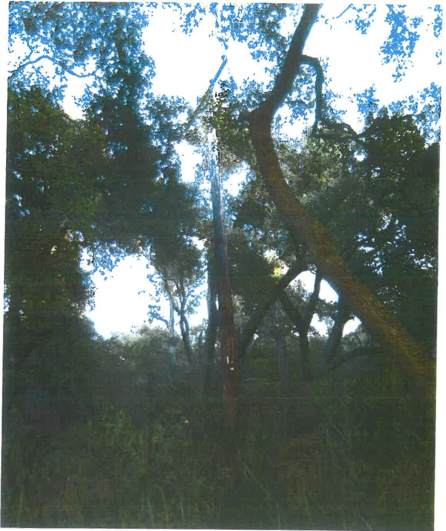
Dist. 49 Deteriorated Pole L / SE
