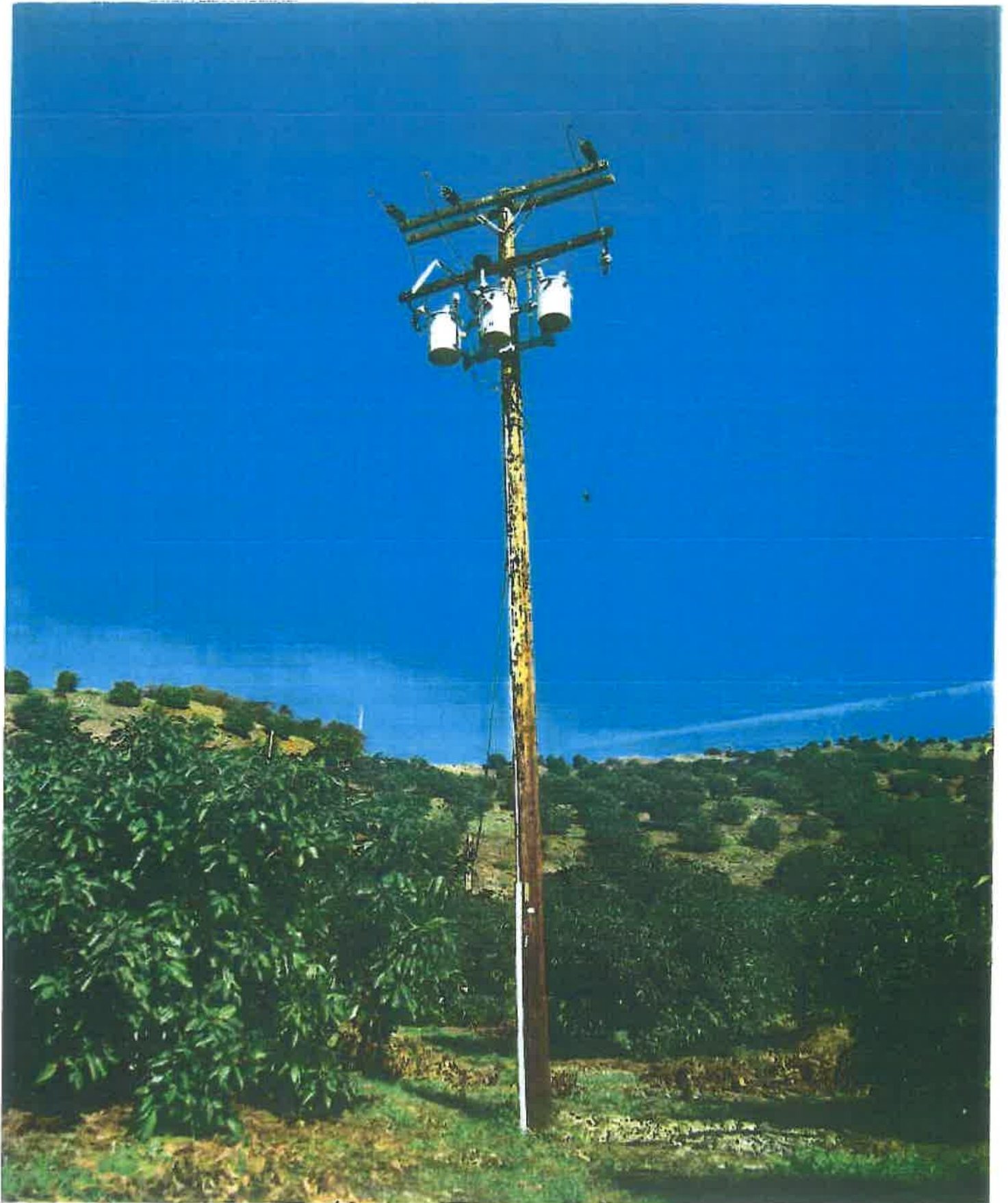
Dist. 49 Deteriorated Pole L / NE
