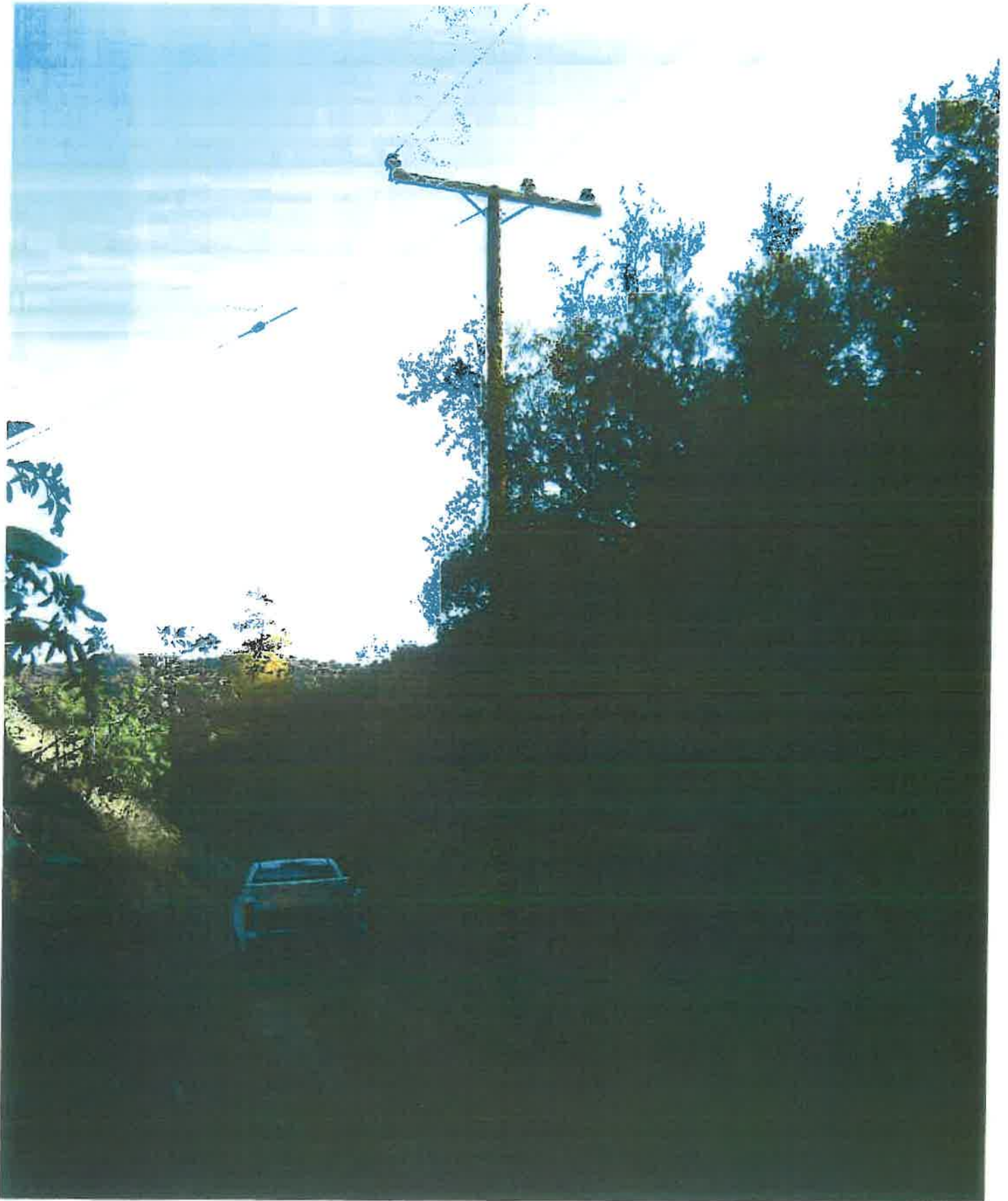
Dist. Deteriorated Pole L / E
