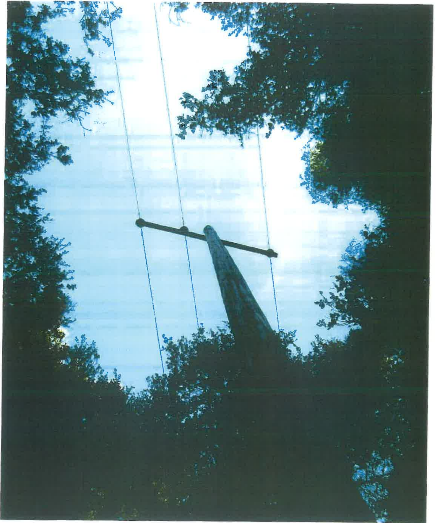
Dist. 49 Deteriorated Pole L / NE
