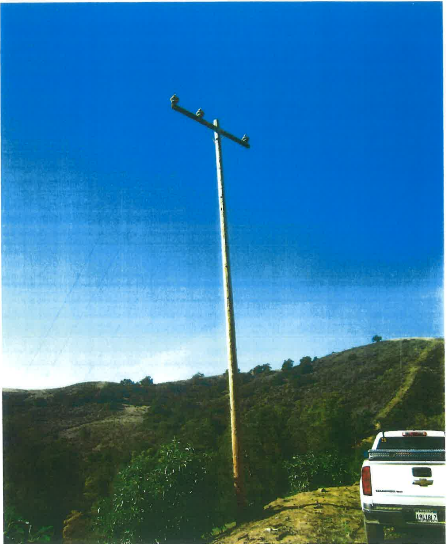
Dist. 49 Deteriorated Pole L / W
