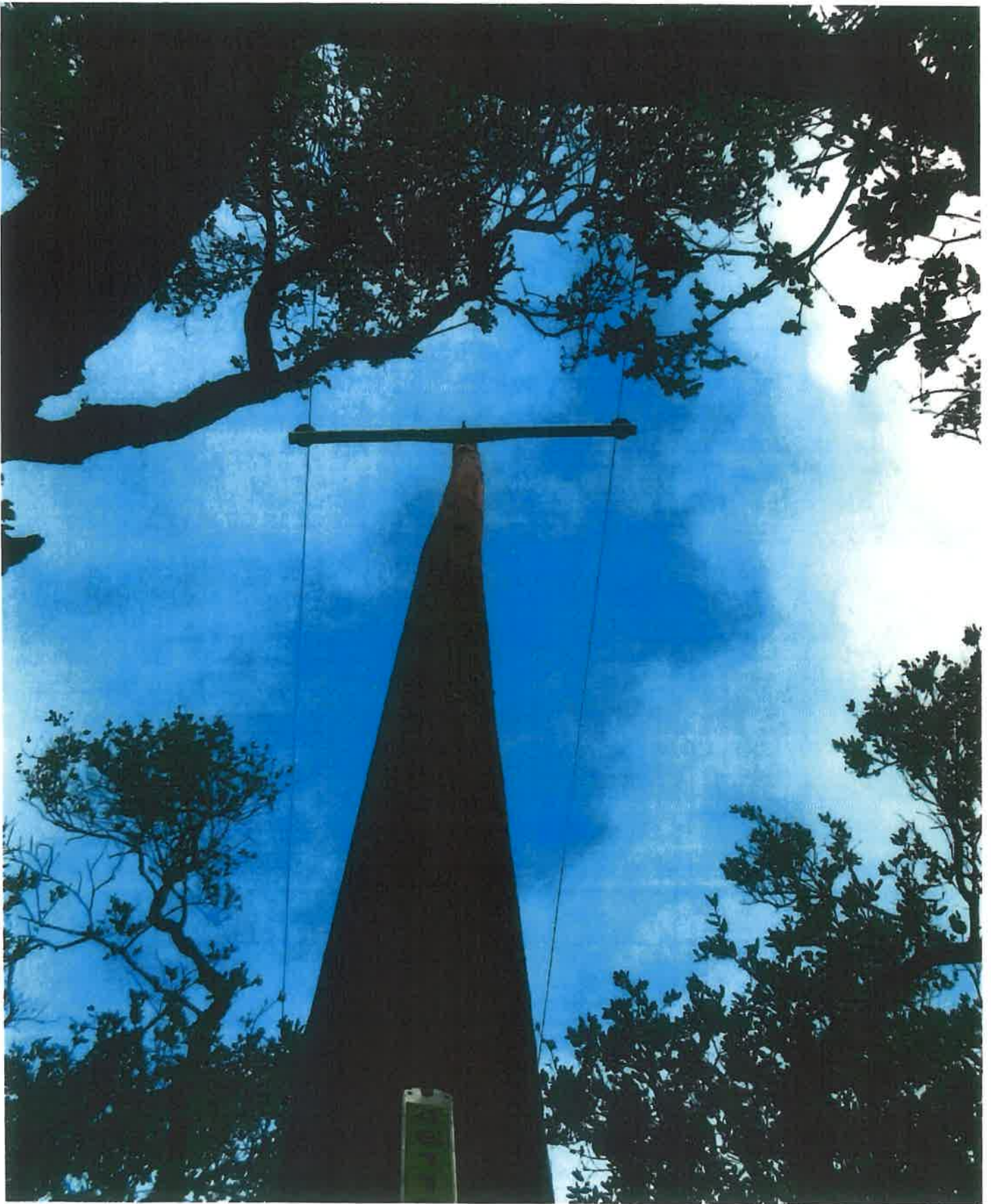
Dist.49 Deteriorated Pole L / N
