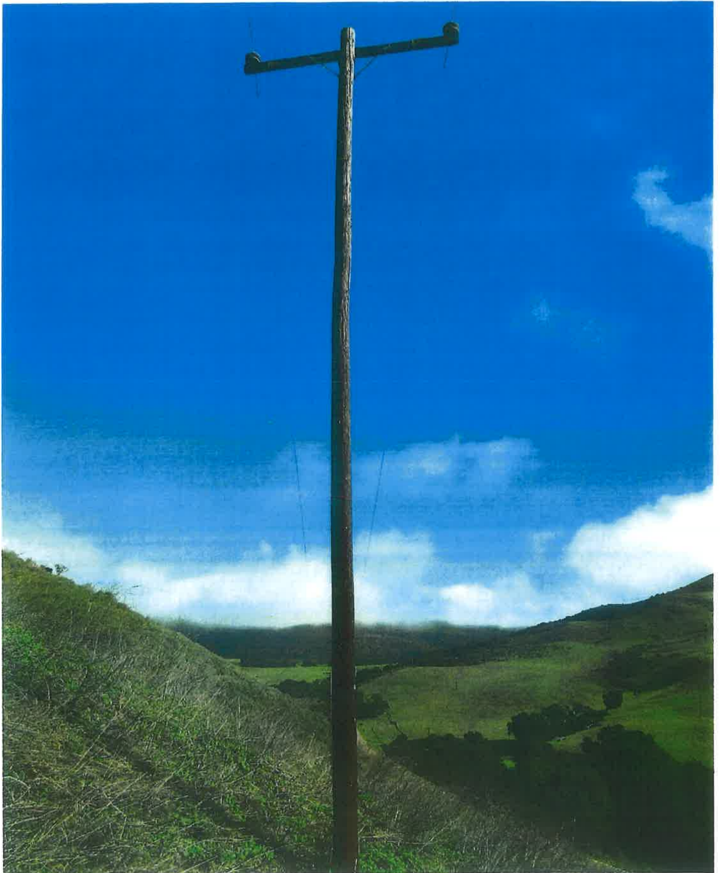
Dist.49 Deteriorated Pole L / N
