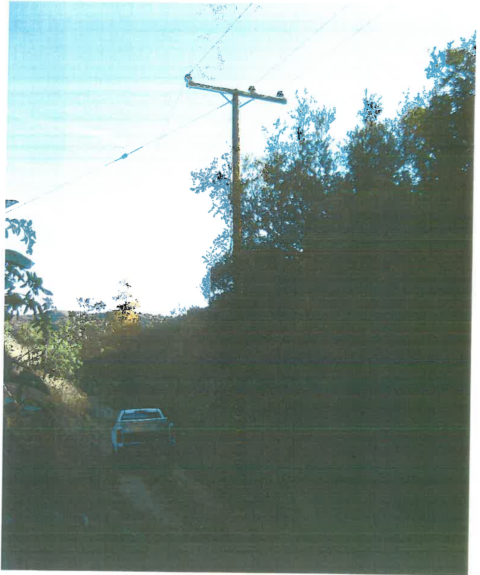
Dist. Deteriorated Pole L / E
