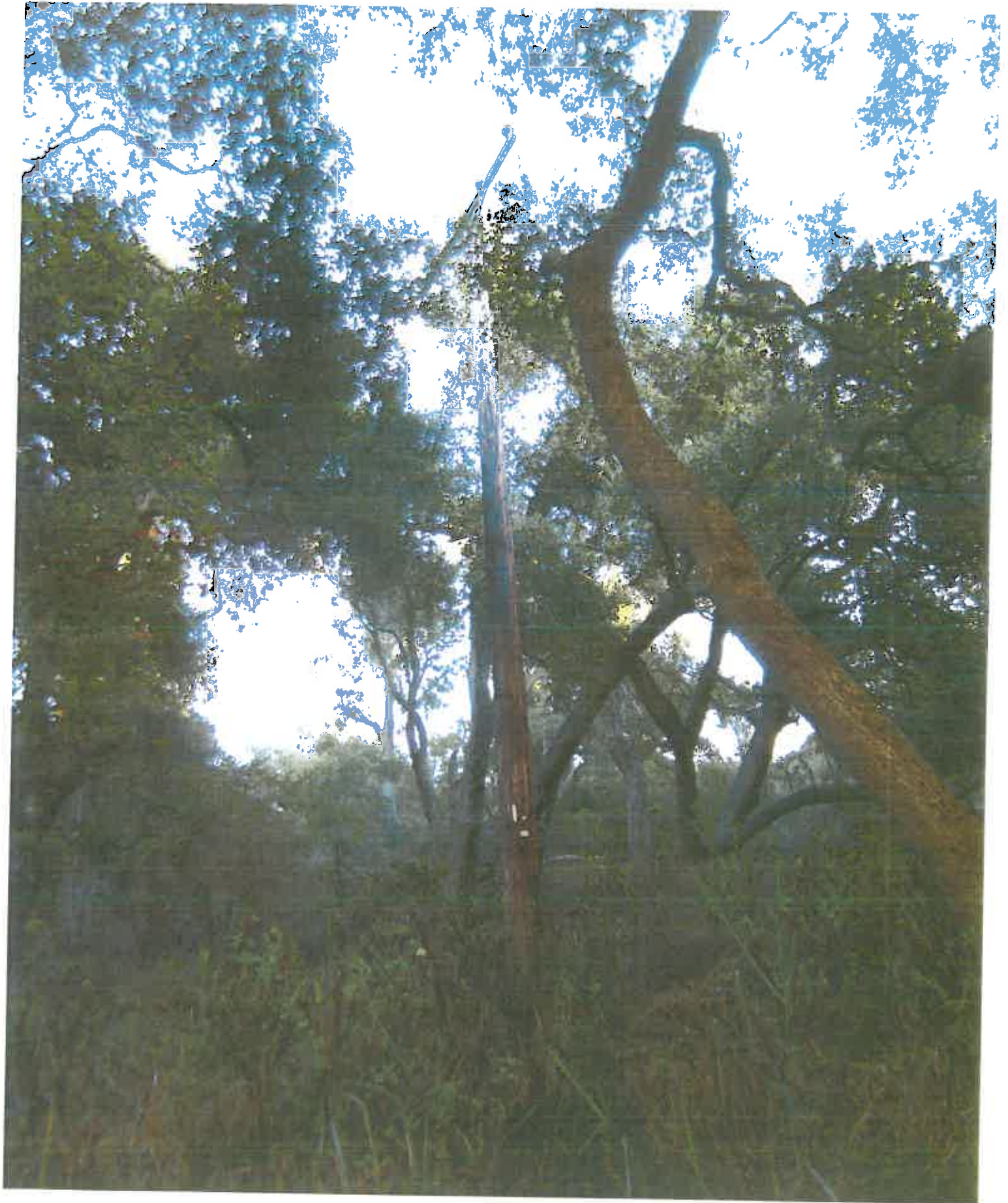
Dist. 49 Deteriorated Pole L / SE
