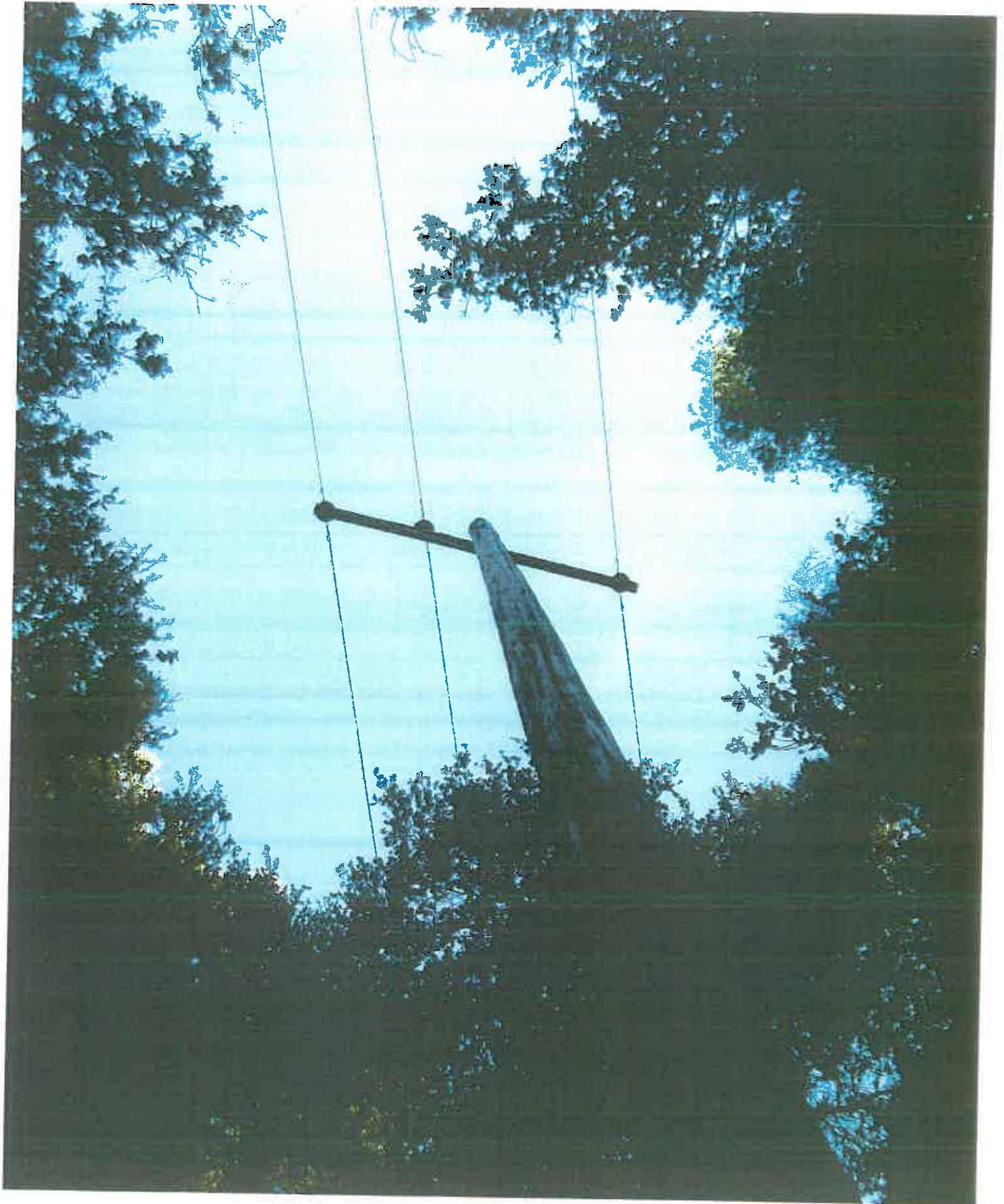
Dist. 49 Deteriorated Pole L / NE
