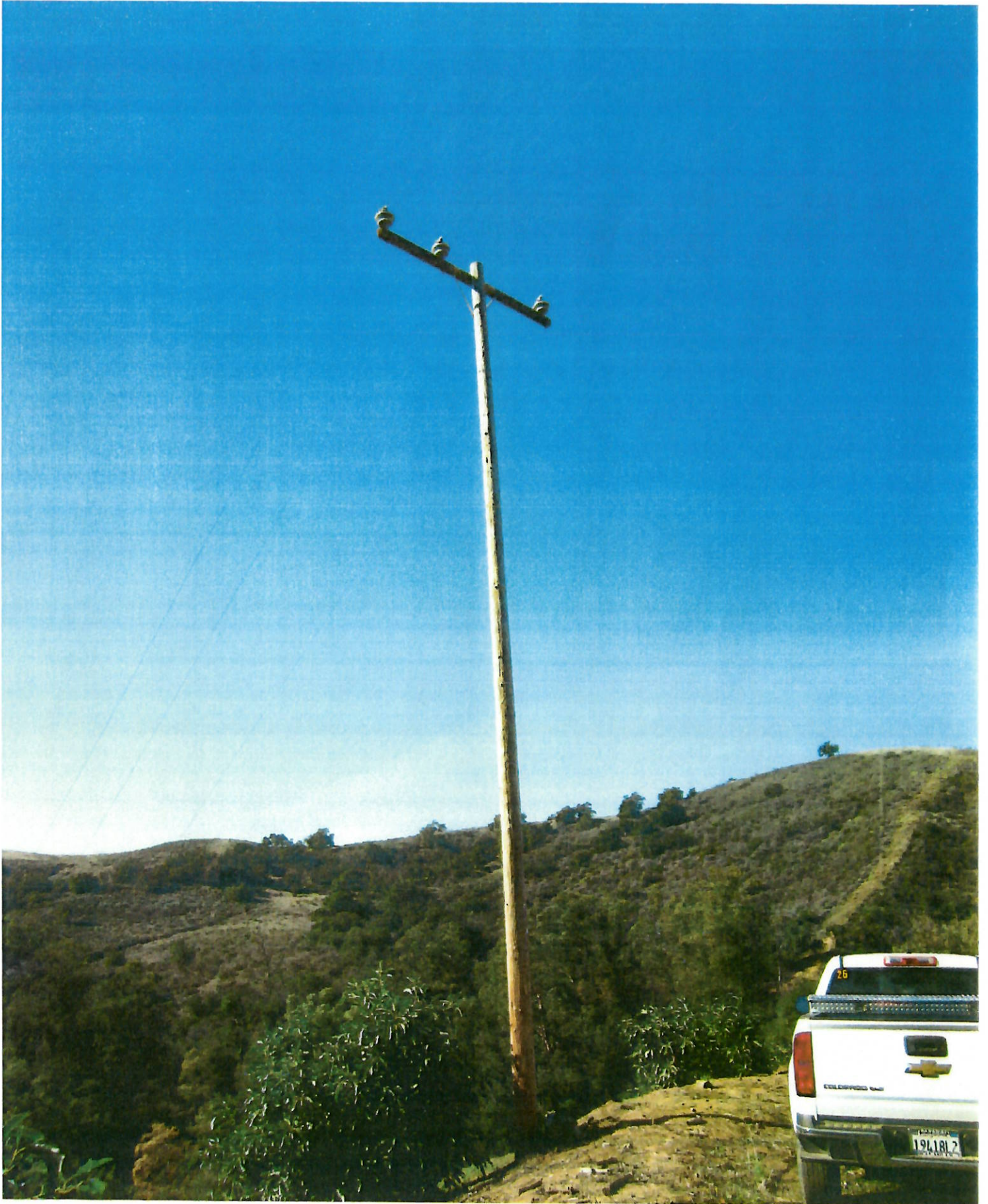
Dist. 49 Deteriorated Pole L / W
