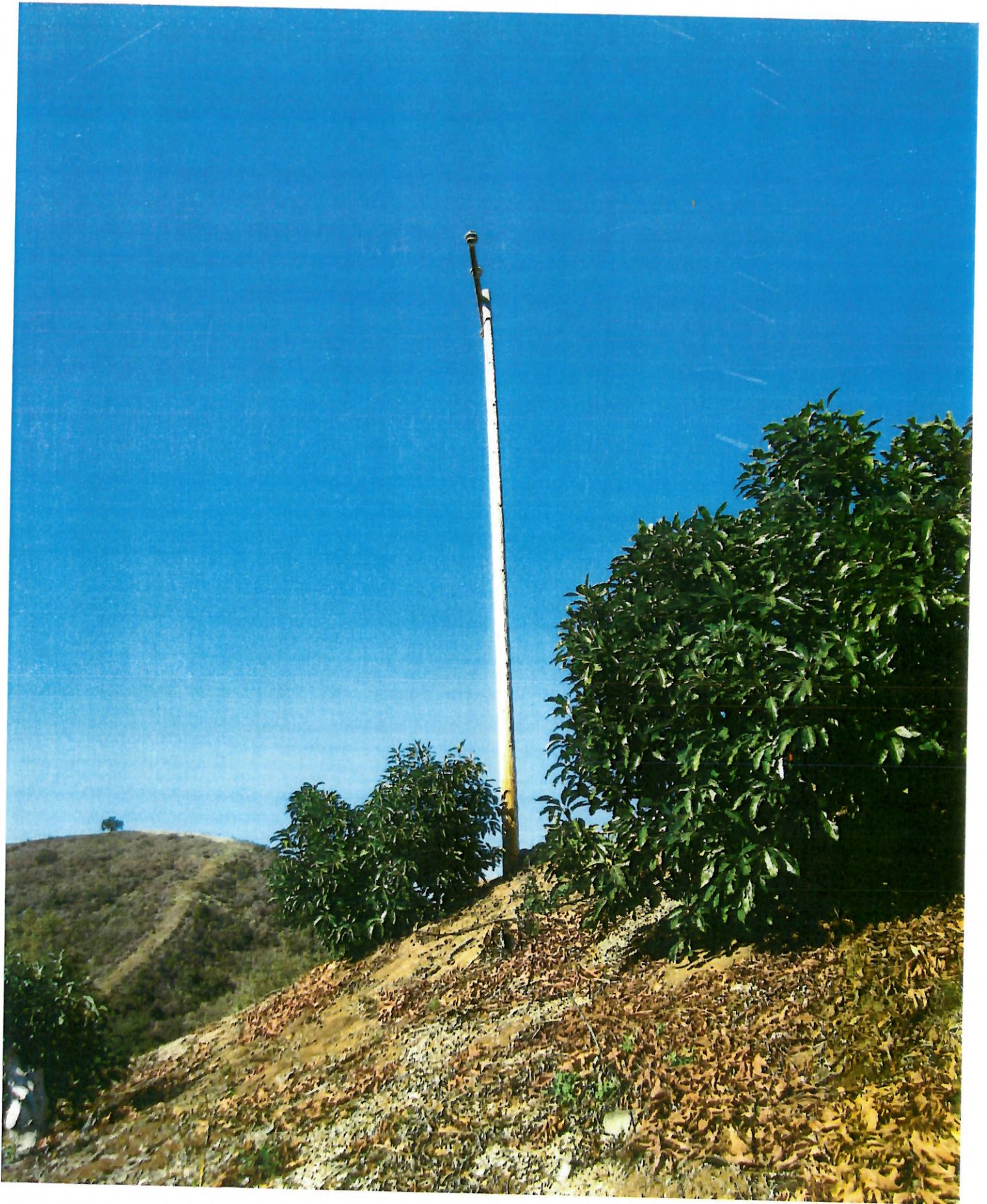
Dist. 49 Deteriorated Pole L / NW
