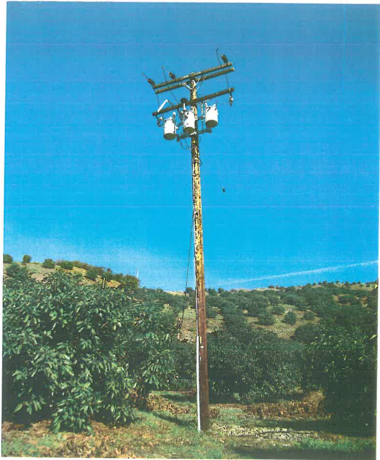
Dist. 49 Deteriorated Pole L / NE
