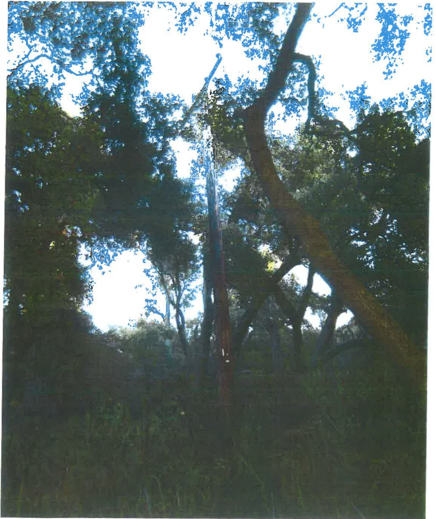
Dist. 49 Deteriorated Pole L / SE
