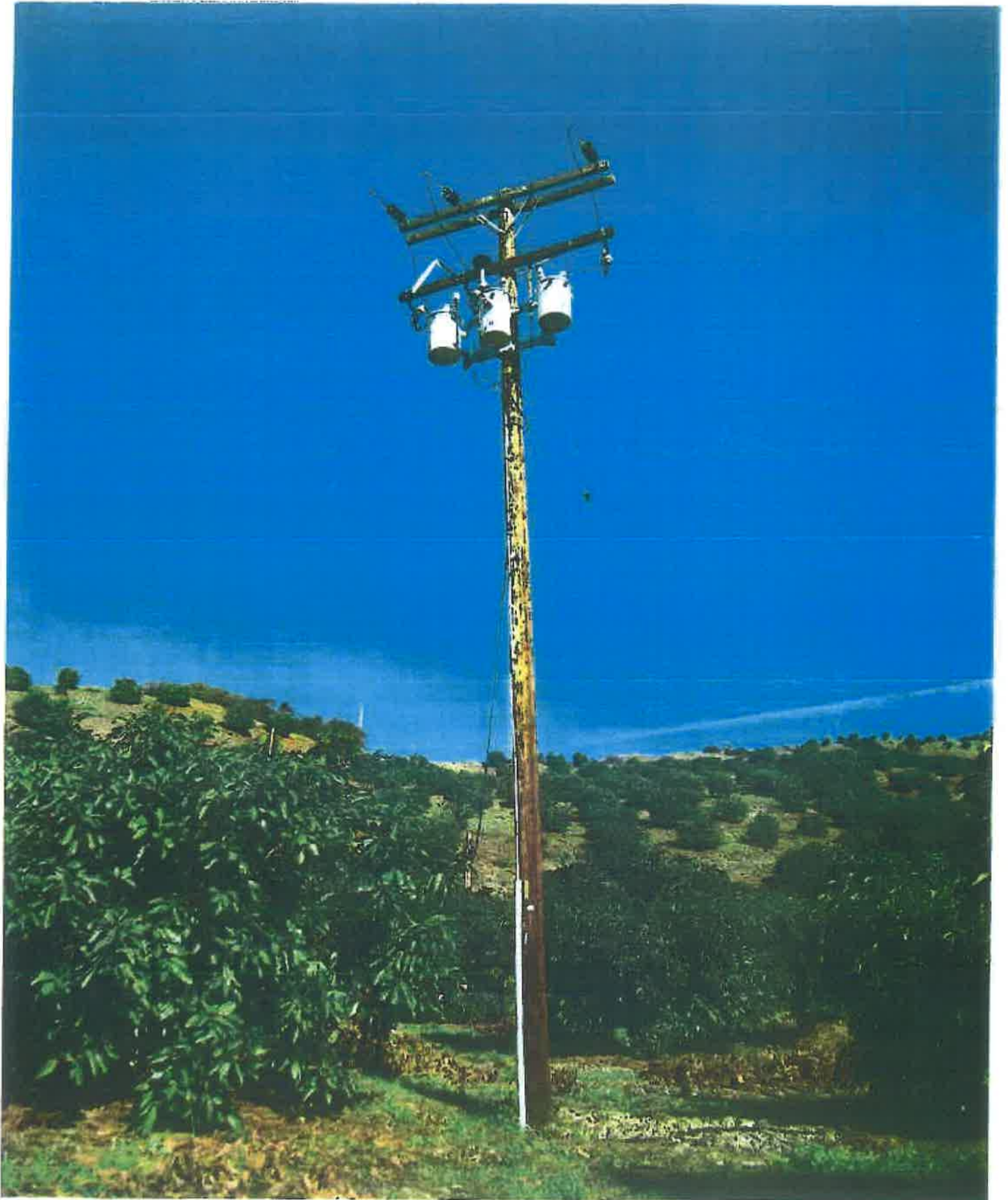
Dist. 49 Deteriorated Pole L / NE
