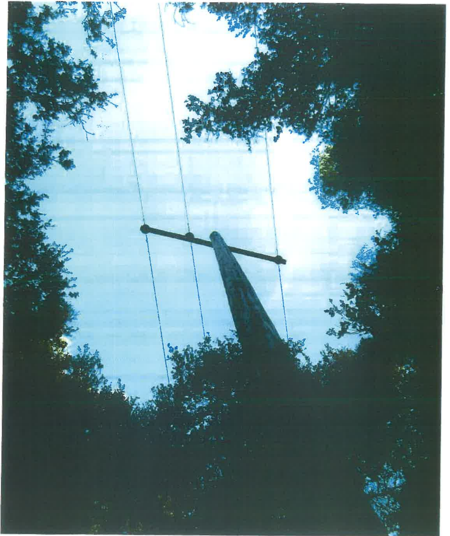
Dist. 49 Deteriorated Pole L / NE
