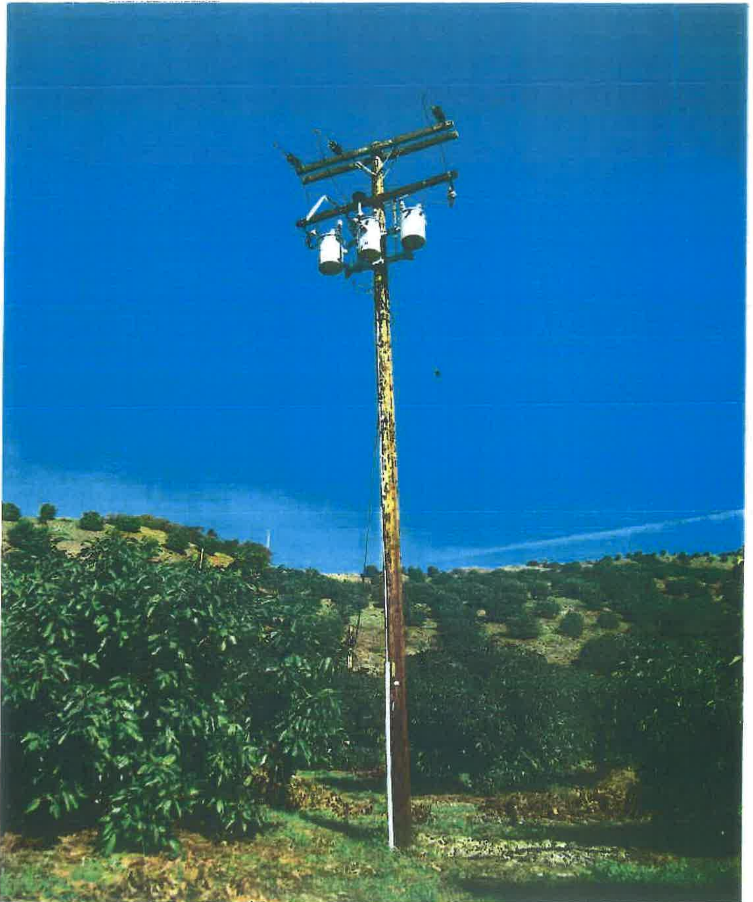
Dist. 49 Deteriorated Pole L / NE
