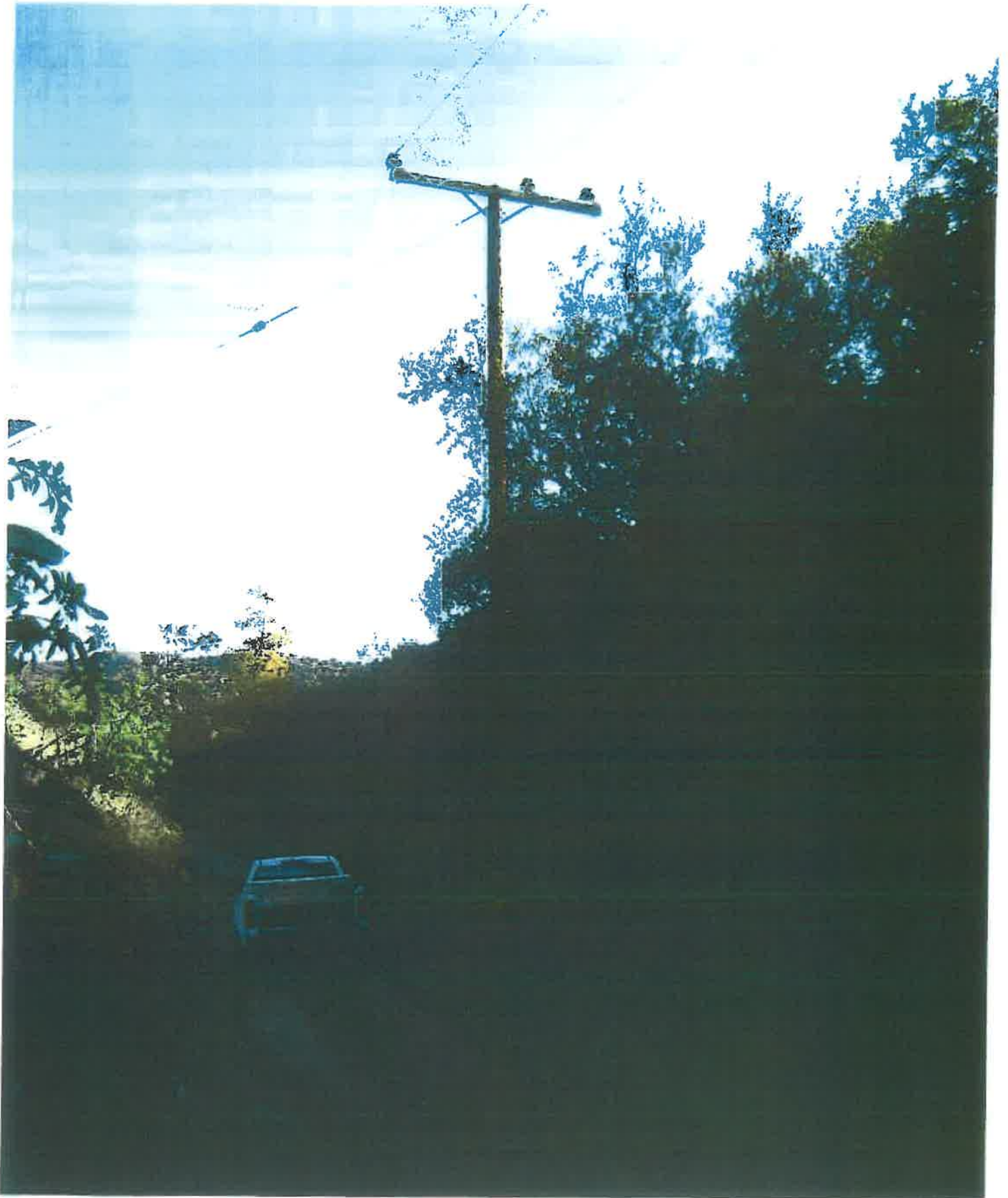
Dist. Deteriorated Pole L / E
