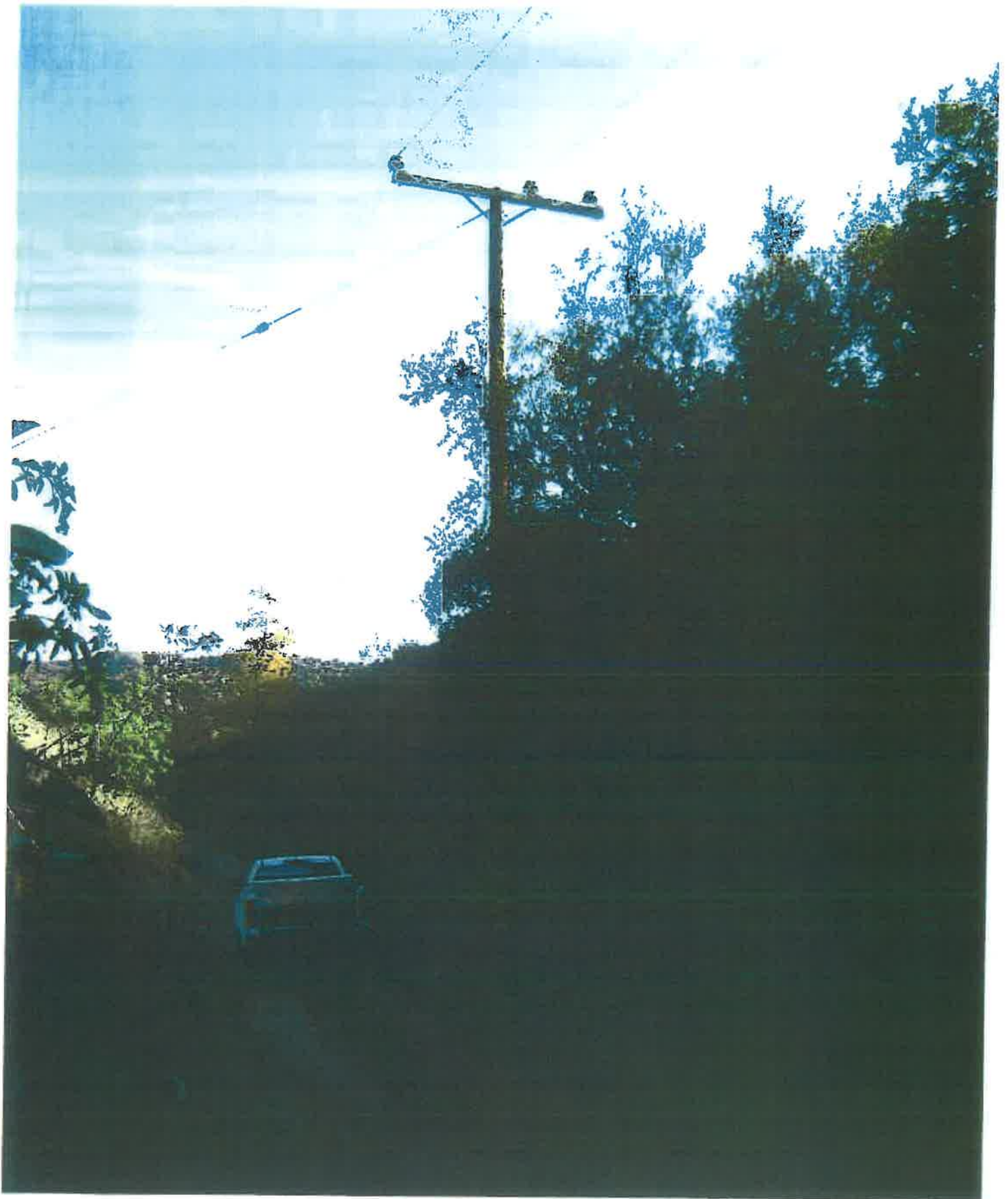
Dist. Deteriorated Pole L / E
