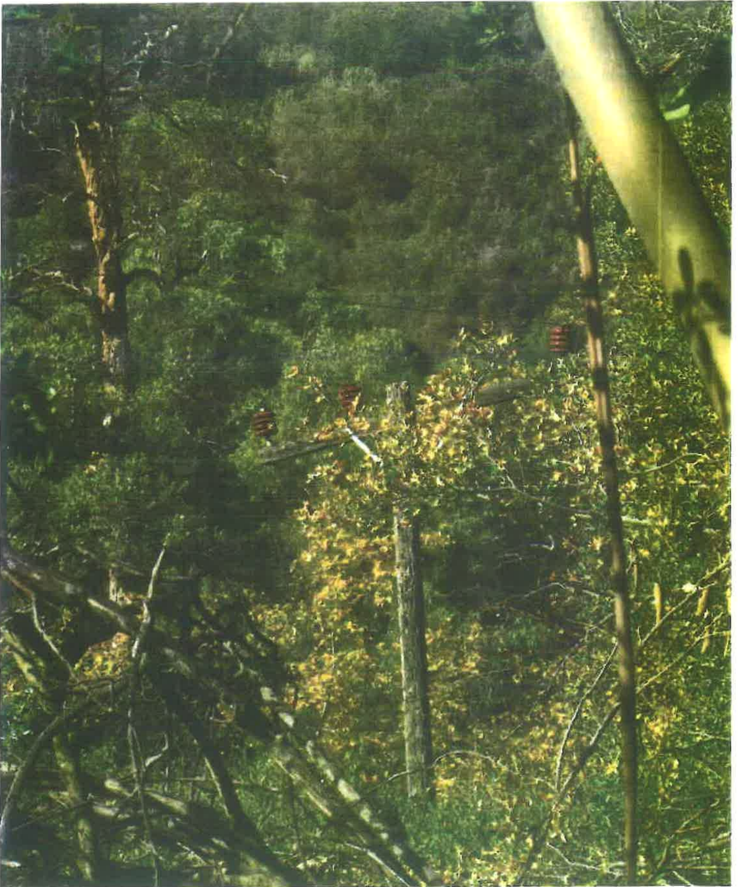
Dist. 49 Deteriorated Pole L / NW
