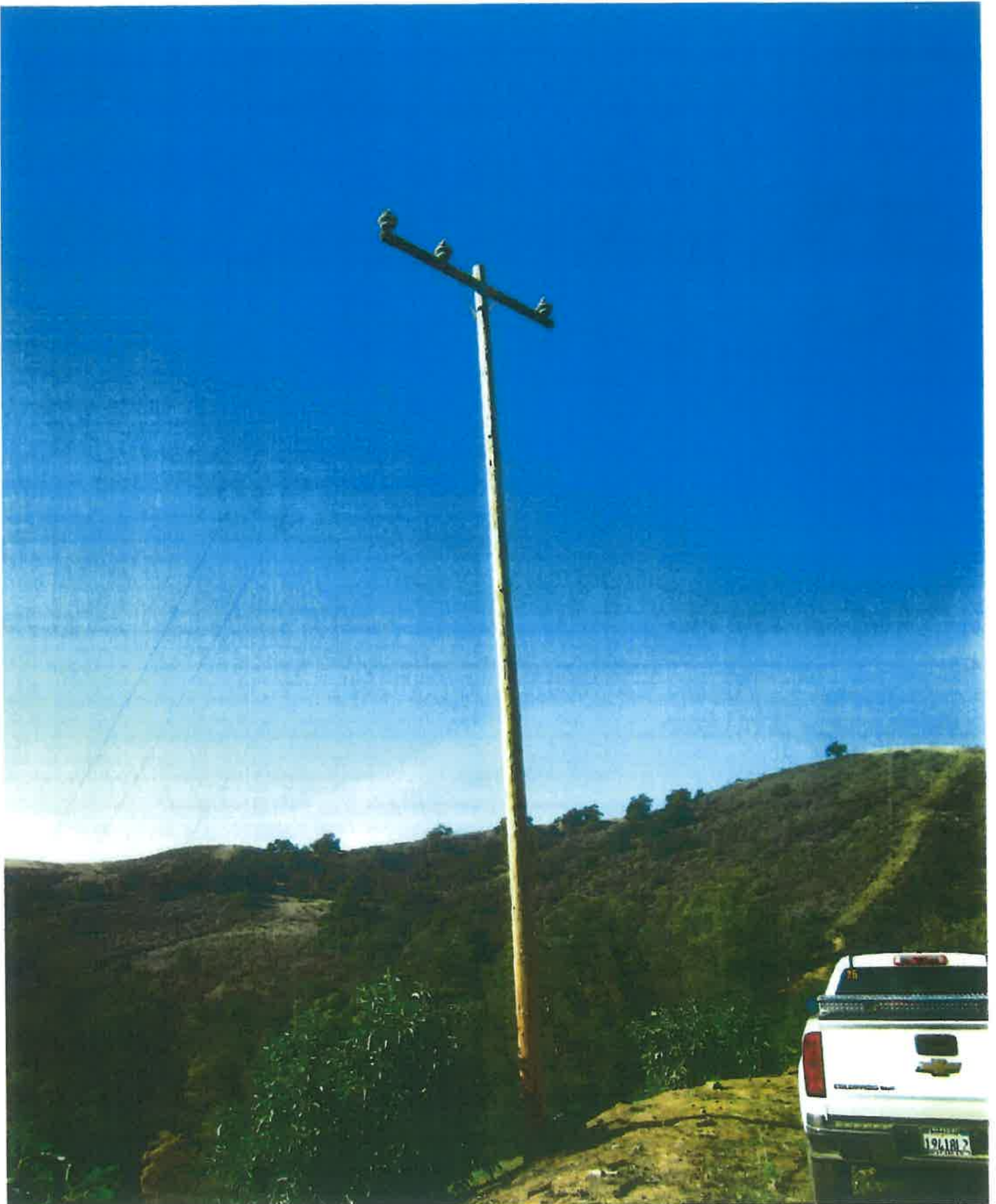
Dist. 49 Deteriorated Pole L / W
