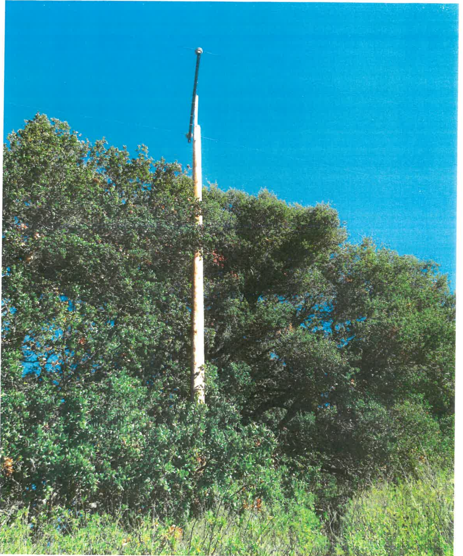
Dist.49 Deteriorated Pole L / N
