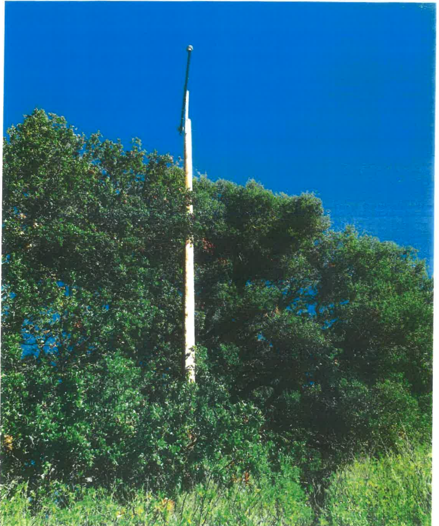
Dist.49 Deteriorated Pole L / N
