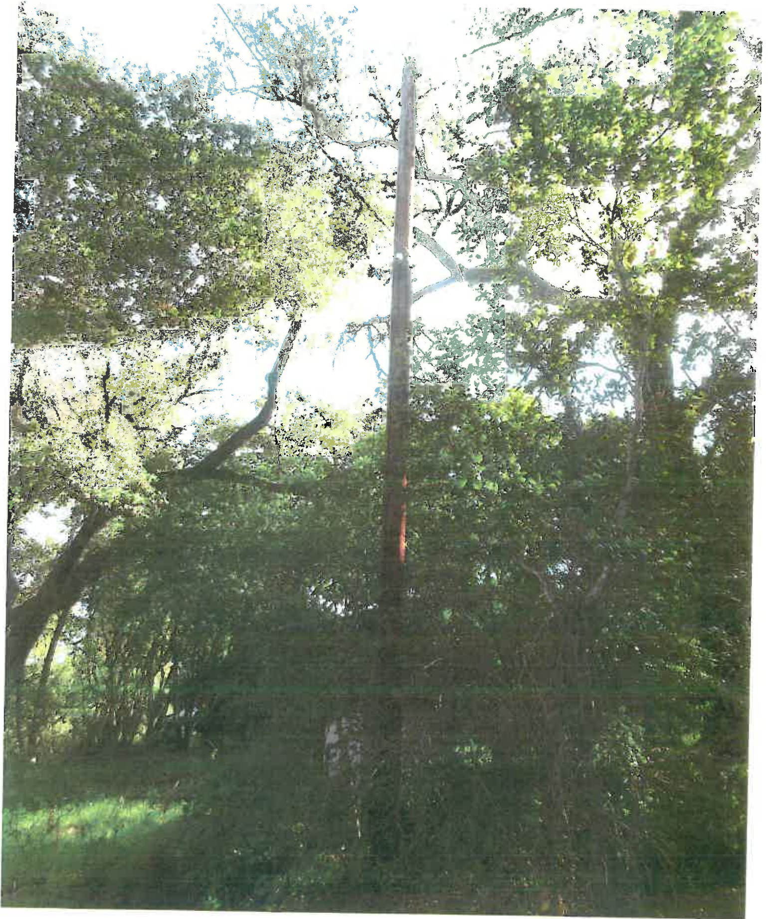
Dist.49 Deteriorated Pole L / E
