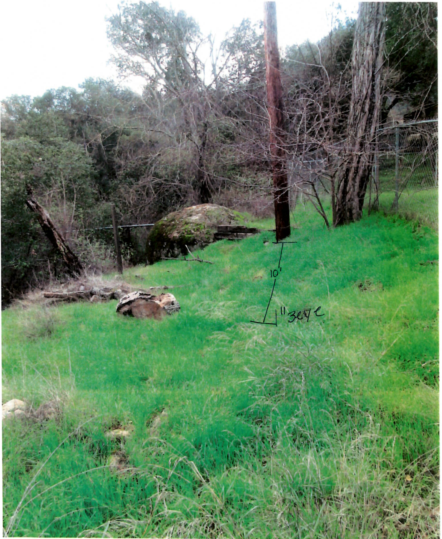
Dist.49 Deteriorated Pole L / S
