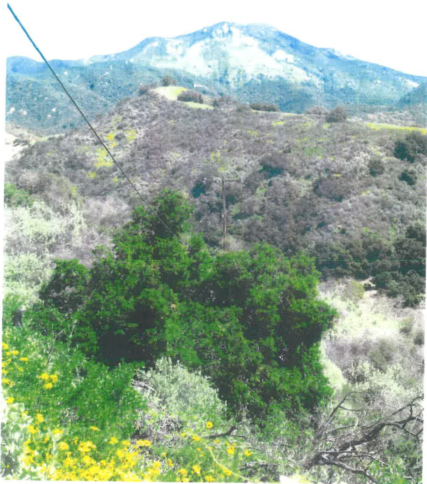
Dist.49 Deteriorated Pole L / NE
