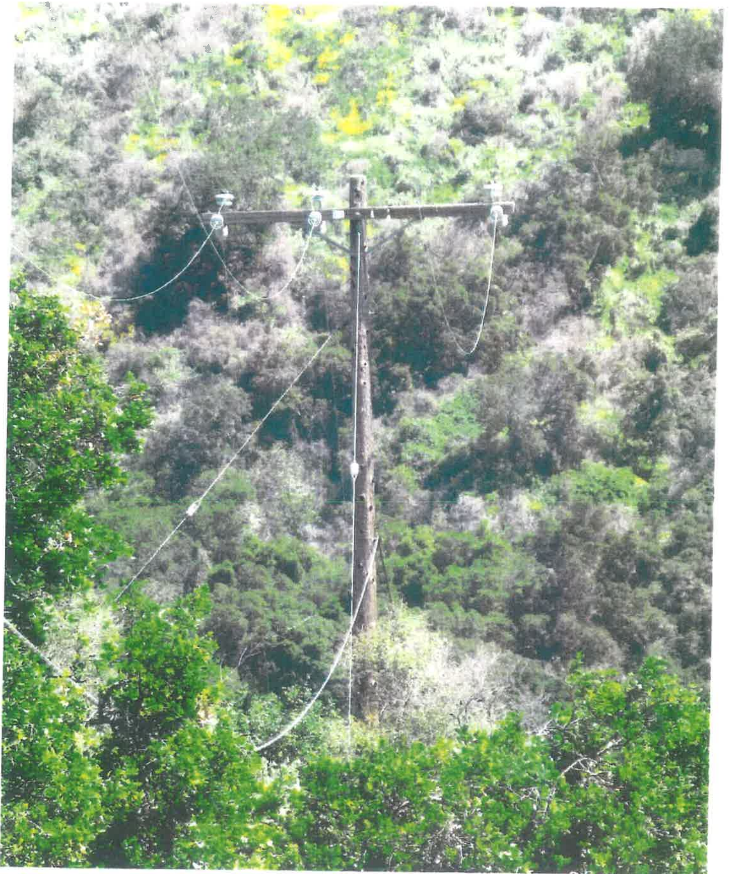
Dist.49 Deteriorated Pole L / NE
