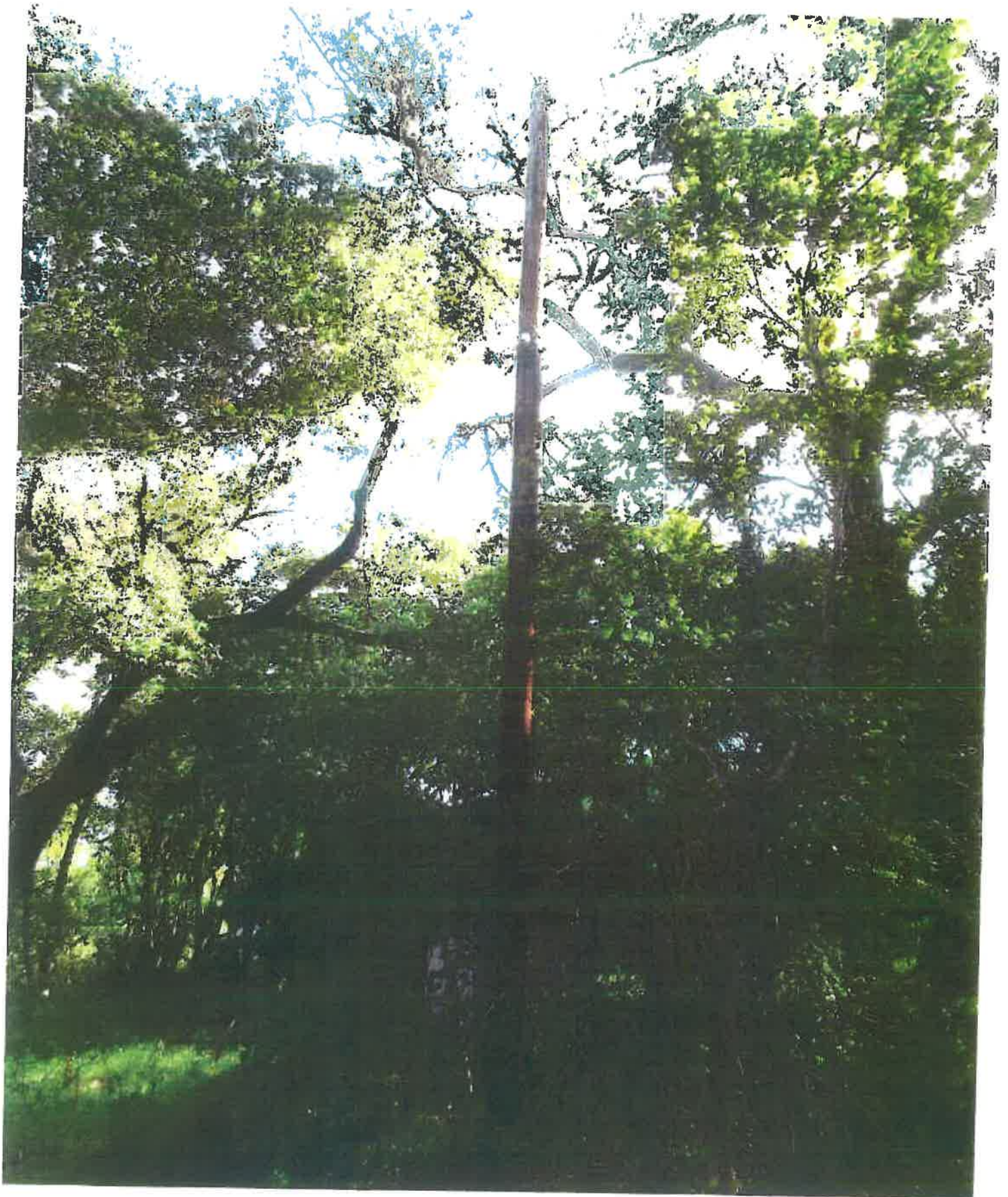
Dist.49 Deteriorated Pole L / E
