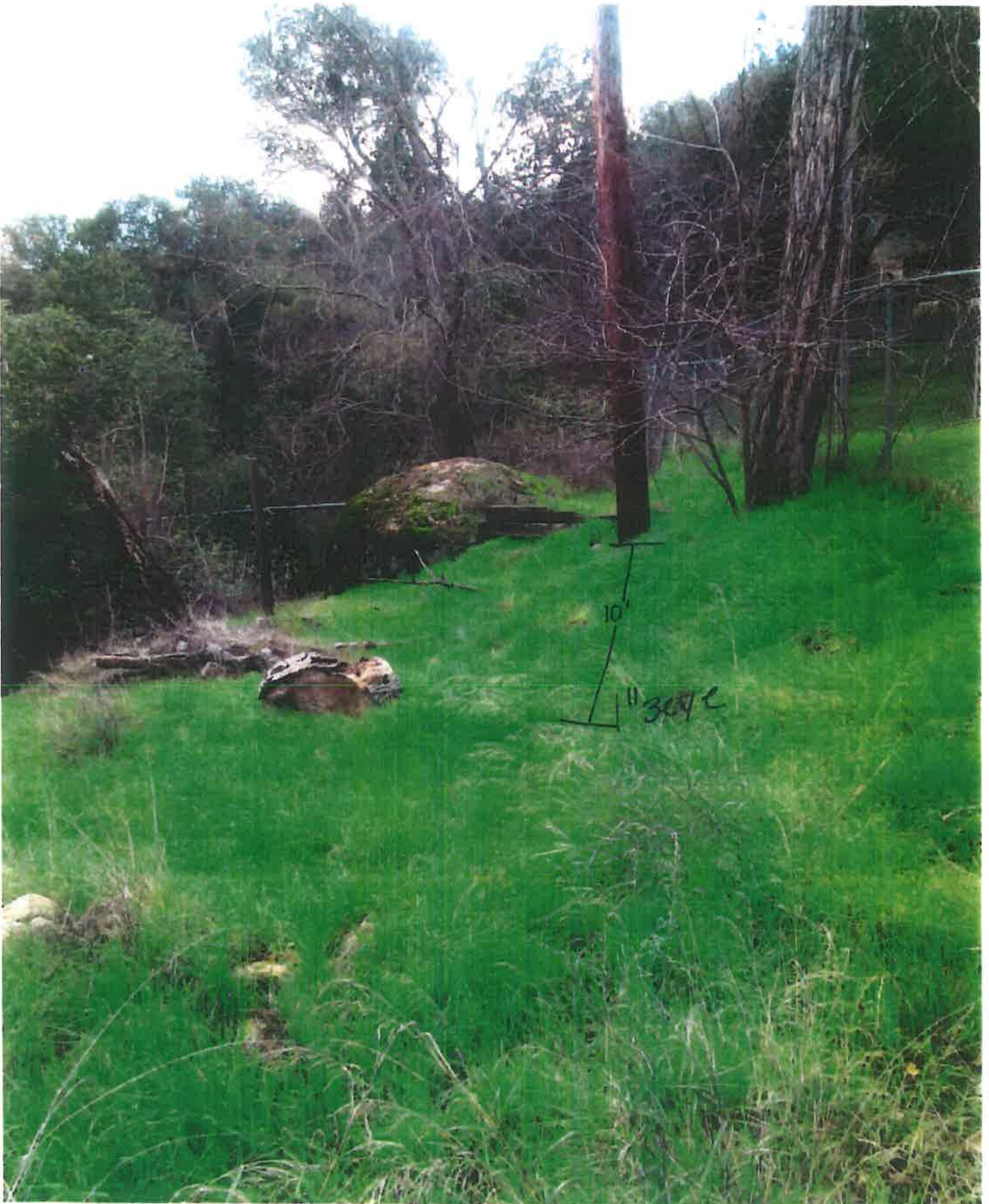
Dist.49 Deteriorated Pole L / S
